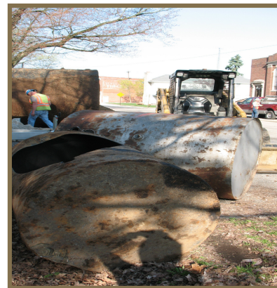
Heating oil and waste oil USTs
