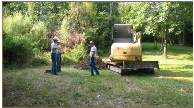
Part of the TPI assessment work involved digging test pits to determine the boundaries of where the landfill waste was buried.
