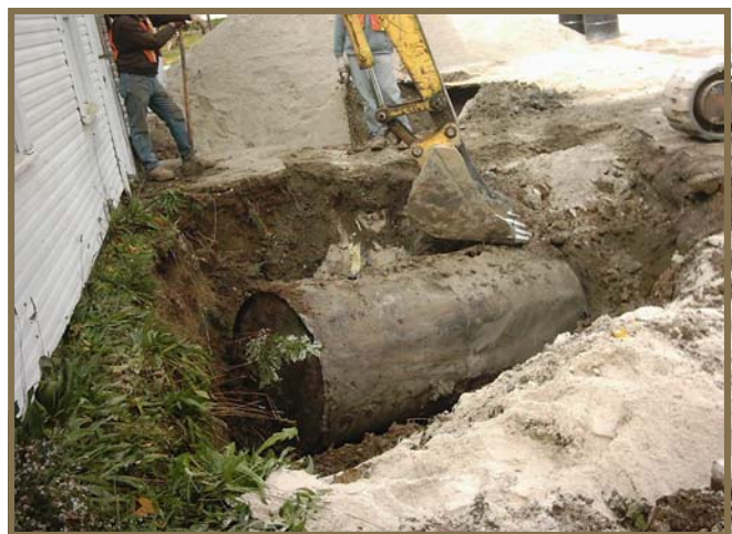
560-gallon gasoline tank
