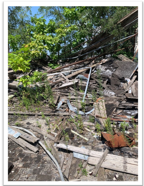
Building Debris Adjacent to Coach Shop
