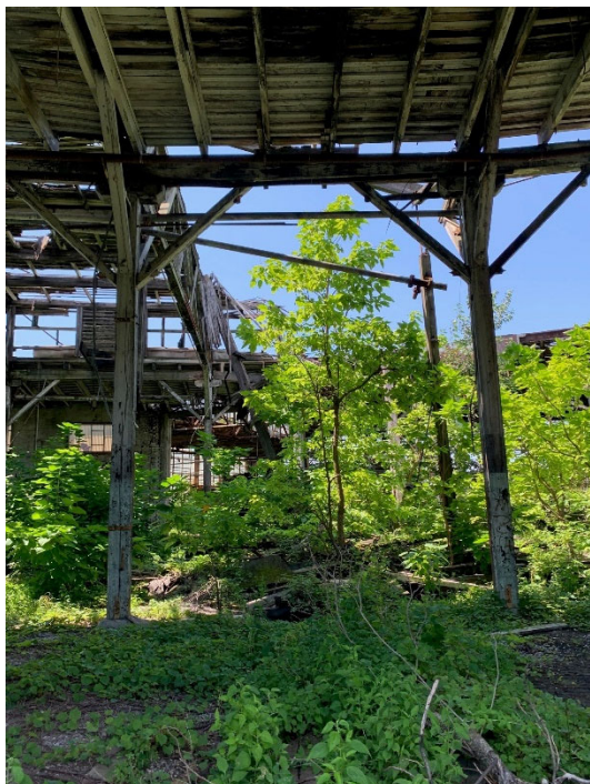
Friable TSI Hanging on Piping
