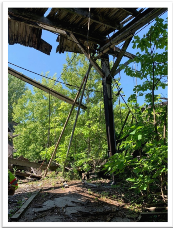
Friable Pipe Insulation in Roundhouse
