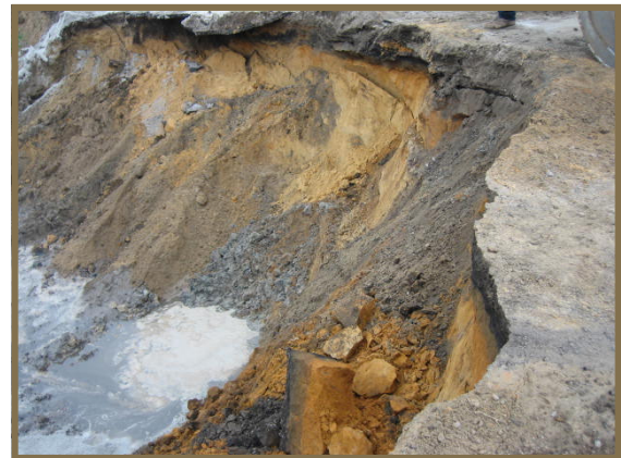
Pit water in excavation
