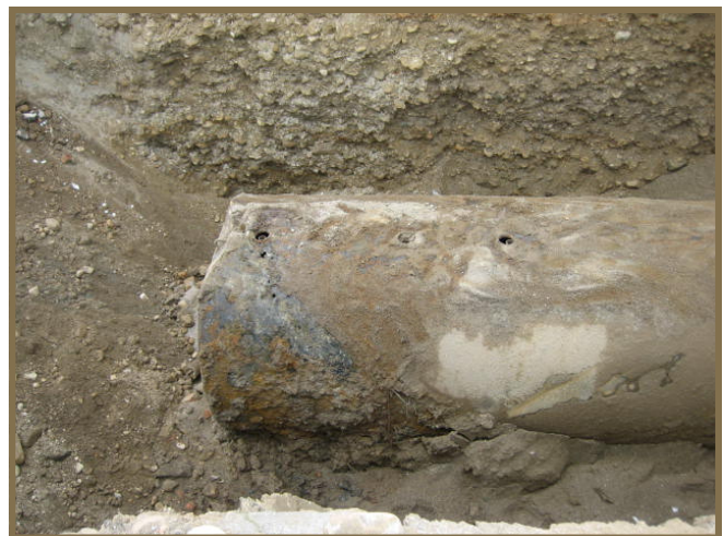
4,000-gallon gasoline underground storage tank
