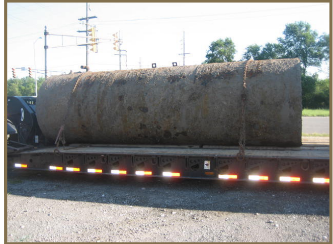
2,000-gallon gasoline underground storage tank
