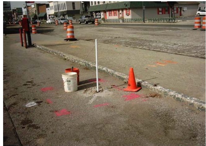
Temporary monitoring well
