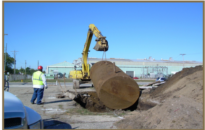
4,000-gallon gasoline tank
