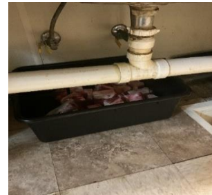
Meat Stored Under Sink
