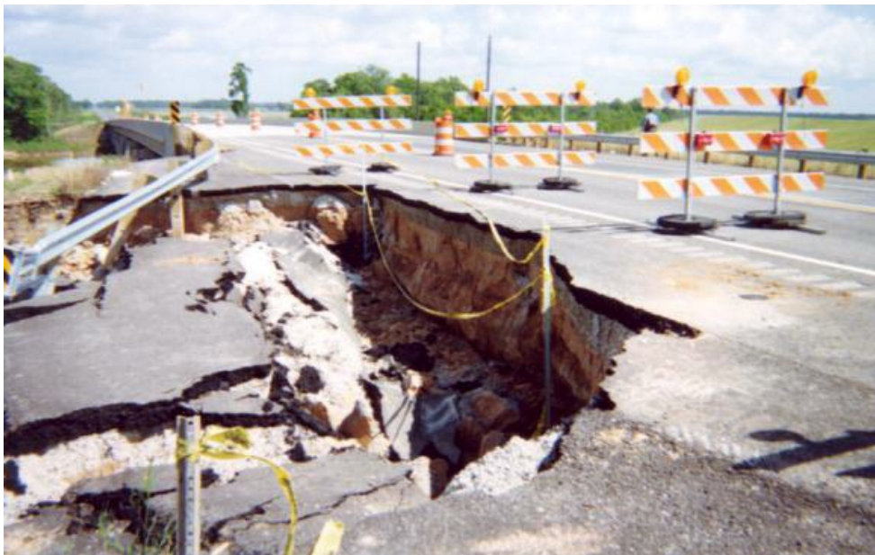
Figure 2- Slope Failure at US-71, Krotz Springs, LA
