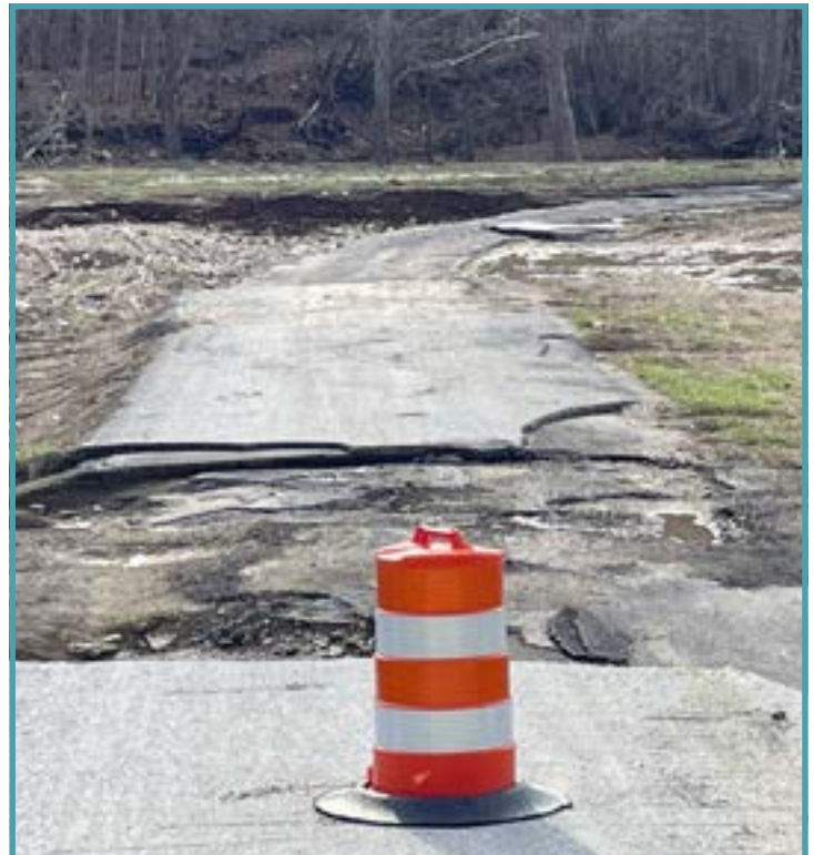
Smith Ridge Road within the floodway of Indian Creek. High velocity water lifted the large piece of asphalt and carried it downstream.
