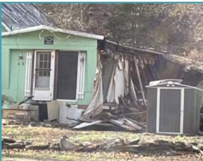
Home damaged on West Fork Indian Creek in Switzerland County.
