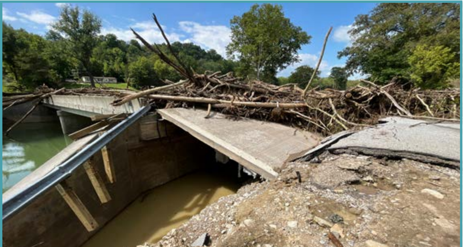
Extensive damage to new bridge construction on Parks Ridge Road over Indian Creek in Switzerland County.
