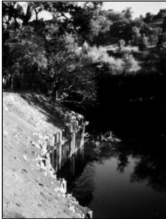
Exhibit 514a: Sheetpile Retaining Wall (Source: NRCS Files)
