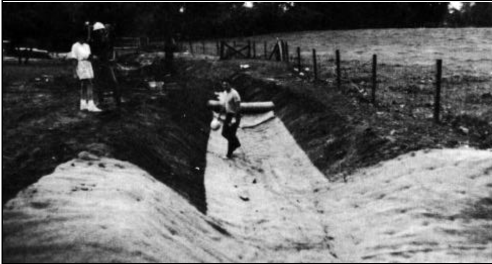
Exhibit 1104b: Proper installation of erosion control blankets in a drainageway (Source: Indiana Erosion Control Handbook)
