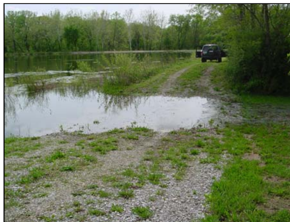
Figure 3-2 Water is starting to overtop this embankment.
