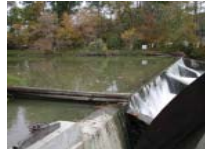
The dam is one of many exterior features that are part of the mill process.
