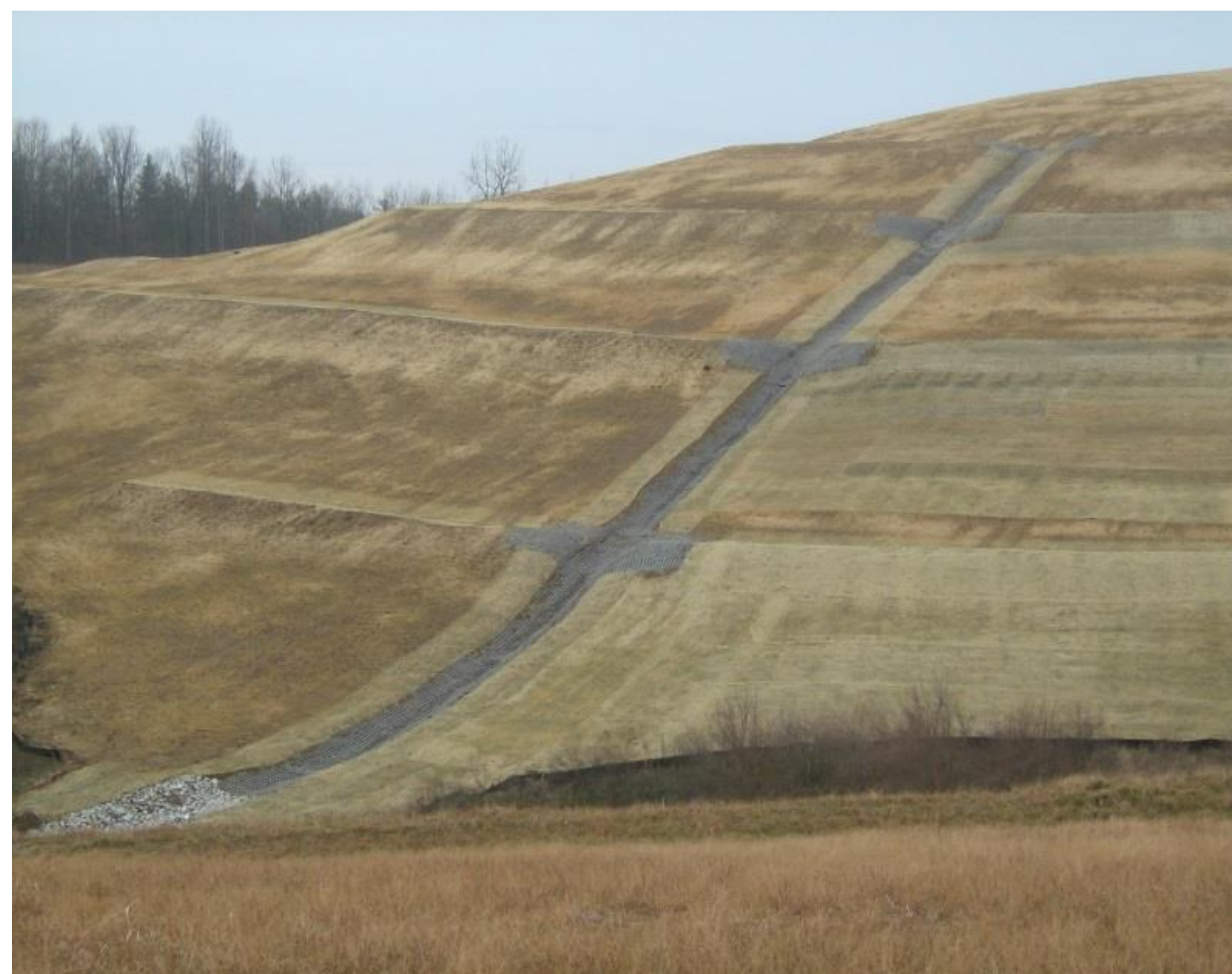
Completed project, south refuse pile, with terracing and installed Flexamat® ditch armoring.
