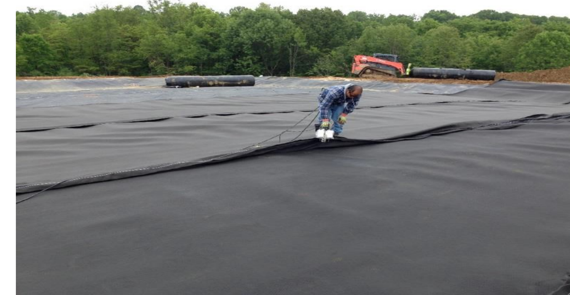
Above: Installed geo-composite drainage layer sections being sewn together, north refuse pile.
