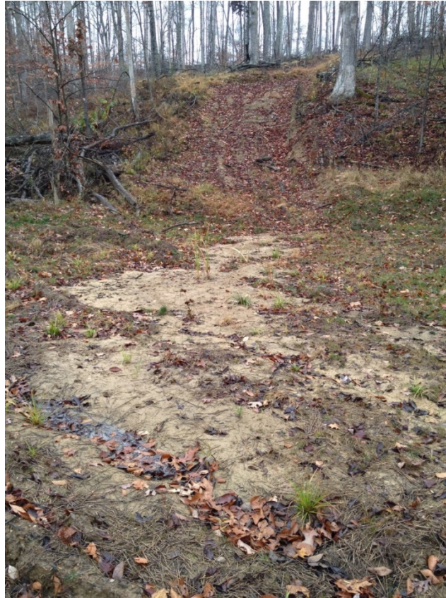
Skid trail not closed out, causing erosion and sediment plume to build up on log yard.
