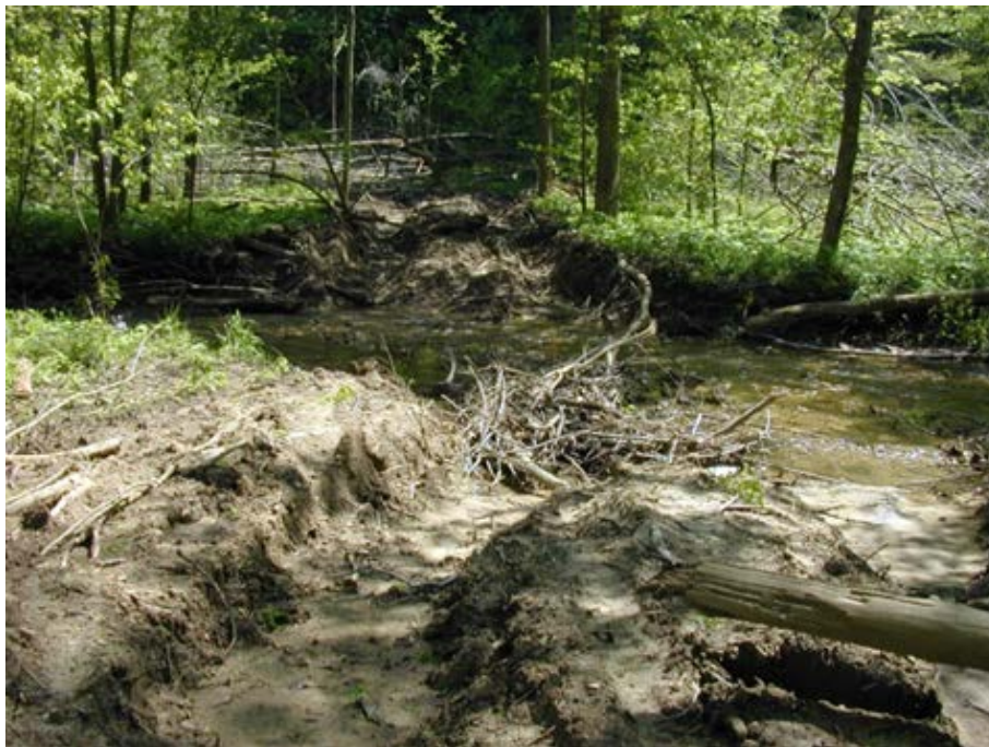
A poorly applied and implemented stream crossing with no attempt to repair.
