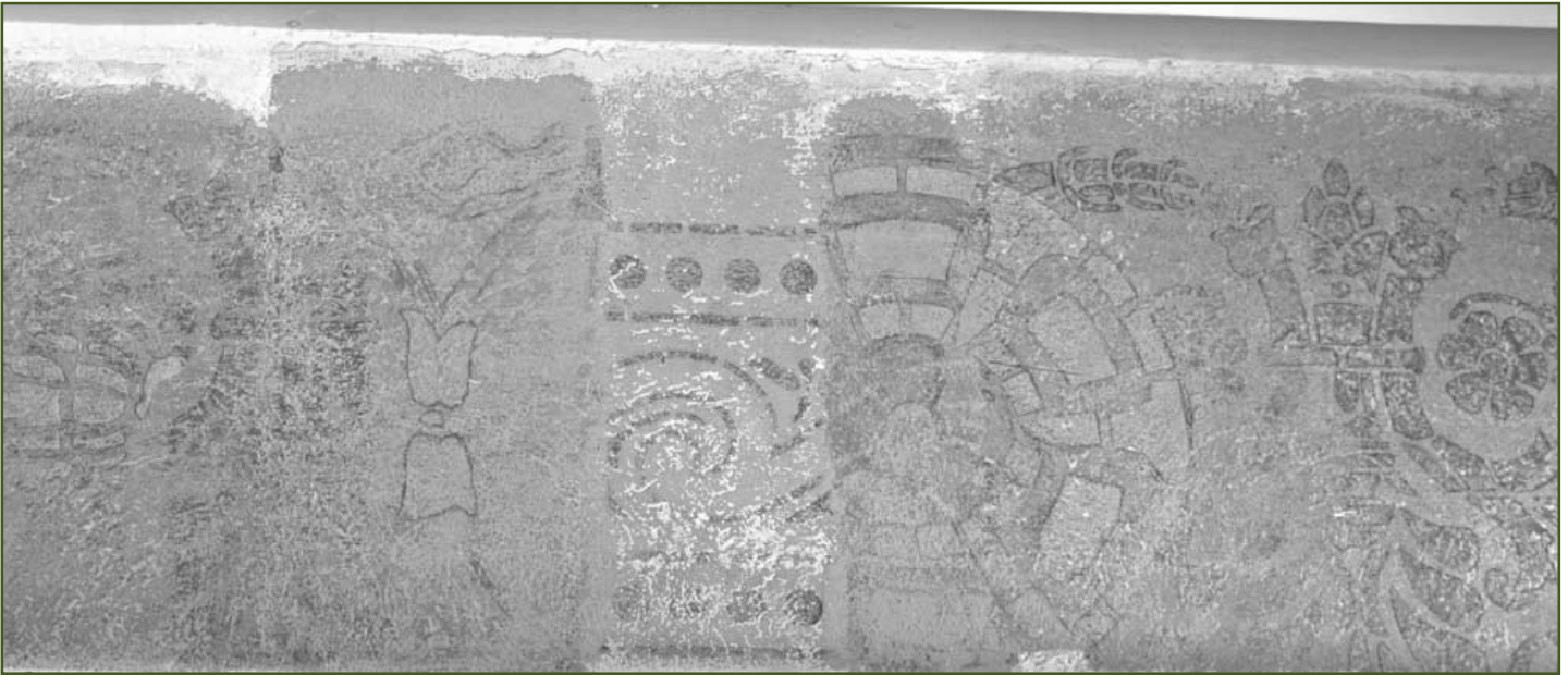
Historical restoration artisans from The Garland Guild uncovered several different paint schemes that have adorned the Library's walls throughout its 118-year history. In 2007, the Supreme Court will restore the Library to its original paint scheme.
