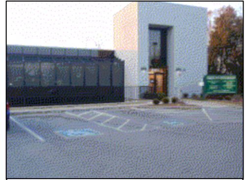
Lack of signs at barrier-free parking
