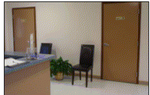
Restrooms with non-compliant signs.
