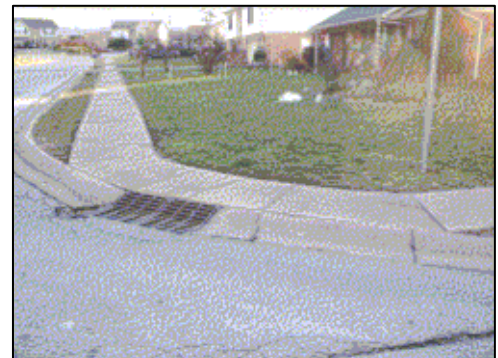
Storm sewer inlet located within area where ramp should be located.
