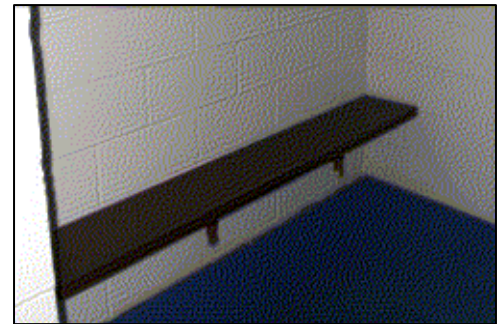
Non-compliant bench in changing area.
