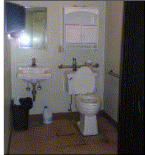
Women’s restroom with non-compliant rear grab bar, no undersink insulation, and lack of space adjacent to toilet for wheelchair.
