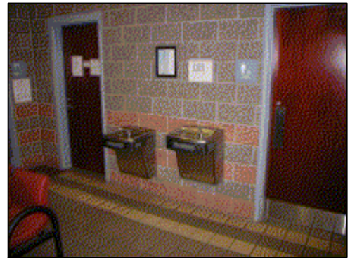
Protruding drinking fountains.
