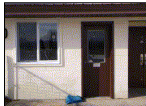
Pool office door has knob hardware.
