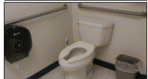
Stall at Animal Control with non-compliant side grab bar, location of toilet flush control, and toilet paper dispenser placement.
