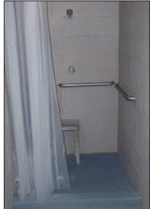
Non-compliant shower threshold.
