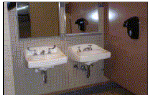
Sinks without proper insulation underneath on hot water and trap.
