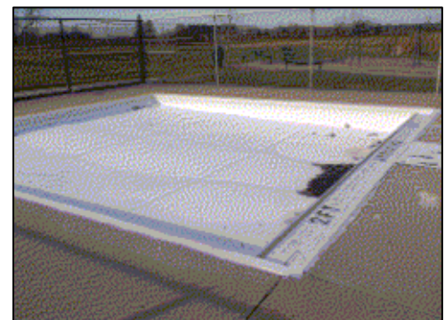
Wading pool does not have access for wheelchair from deck.
