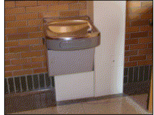
Non-compliant drinking fountain.
