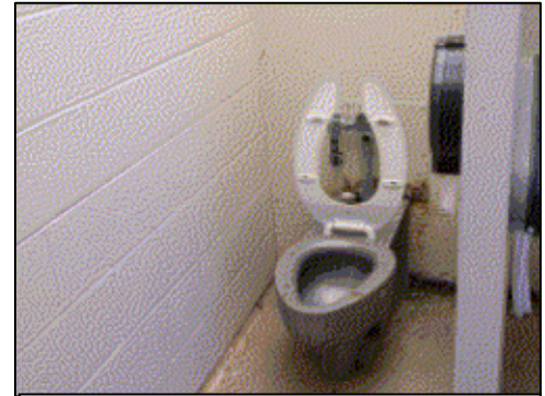
Non-compliant restroom stall at Gresham Park.
