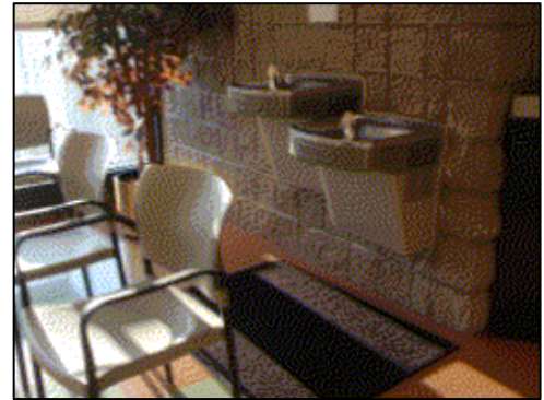
Lack of clear space at Health Department drinking fountain.
