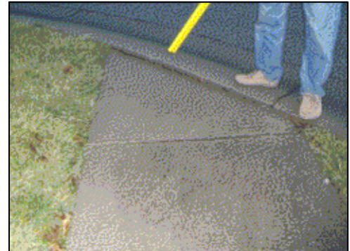
Sidewalk with displacement at curb and lack of curb ramp.
