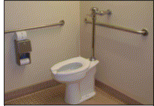
Flush valve on narrow side of toilet.
