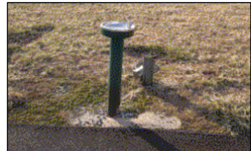
Inaccessible drinking fountain provides no knee space below.
