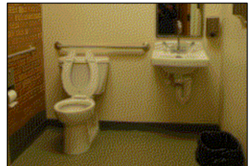
Restroom with sink in required clear area adjacent to toilet.
