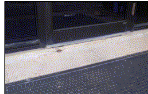
Non-compliant height threshold.
