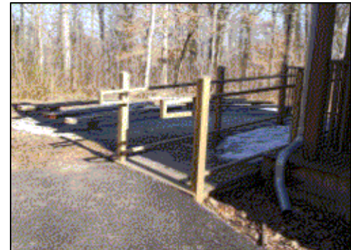
Protruding wood ramp handrail extension at Battle of Corydon Park.
