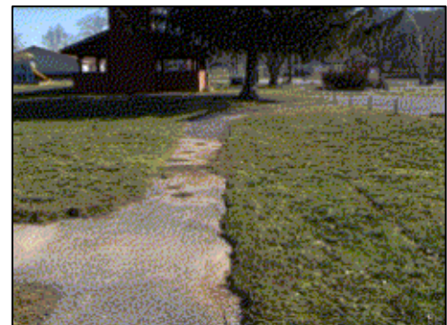
Non-compliant route from parking and shelter to restrooms.
