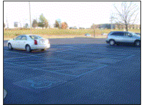
Justice Center barrier-free parking lacks proper signage.
