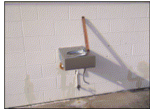
Non-compliant drinking fountain.
