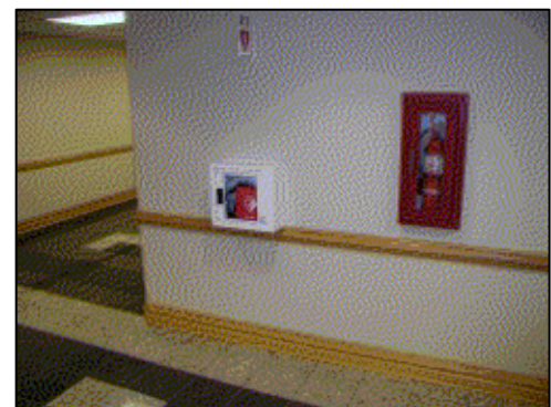
Protruding defibrillator in hallway.
