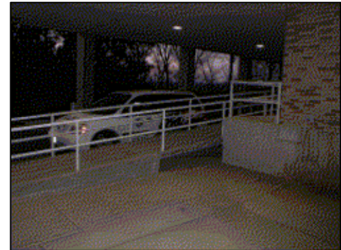
West ramp lacks edge protection.
