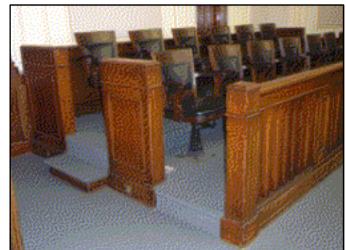
Jury box is not accessible.
