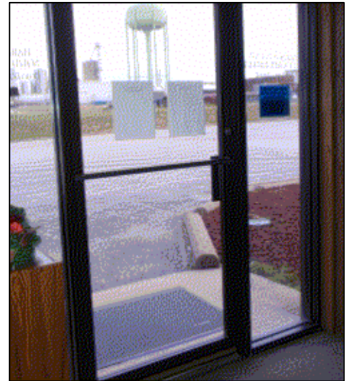
Front entry door to Solid Waste has glazing that is breakage hazard.
