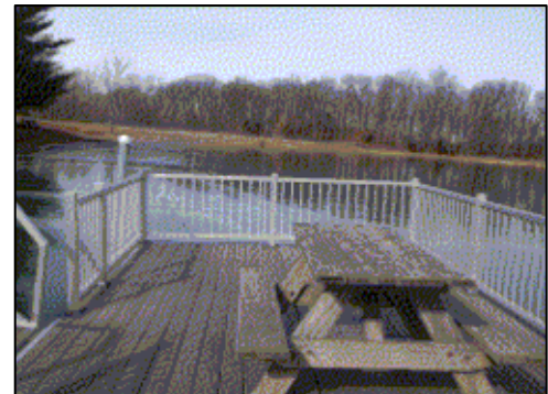
Fishing pier provides no areas of lowered railing for wheelchairs.
