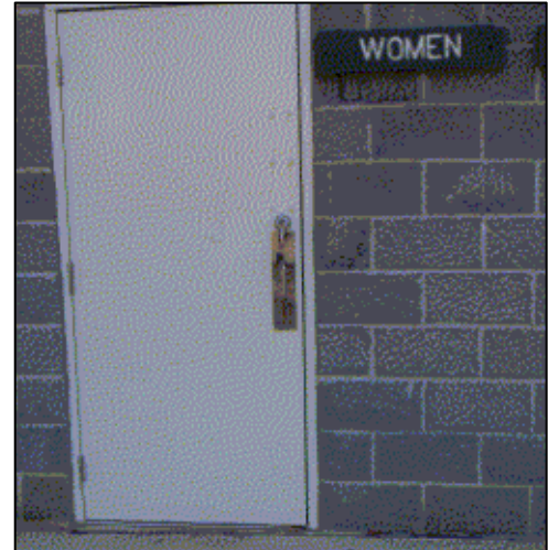
Non-compliant restroom signage.
