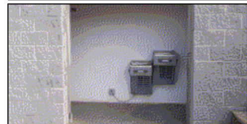
Non-compliant drinking fountains at press box restrooms.
