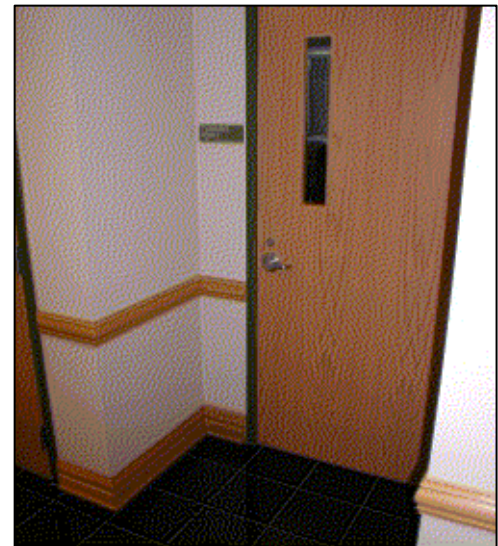
Inadequate latch side space at door.
