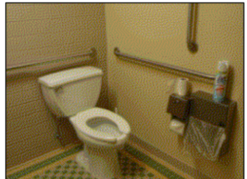
Proper 48" length side grab bar mounted too close to rear wall.
