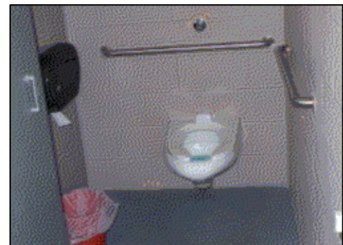
Non-compliant stall has in swinging door, and toilet paper dispenser and trash block access to inadequate clear space.
