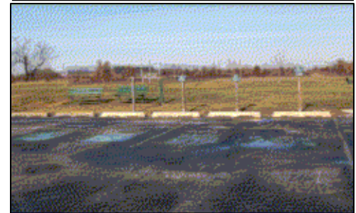
Barrier-free parking has no access aisles and signs are too low.
