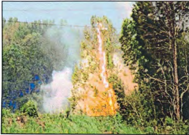
Direct contact can cause flashovers.
