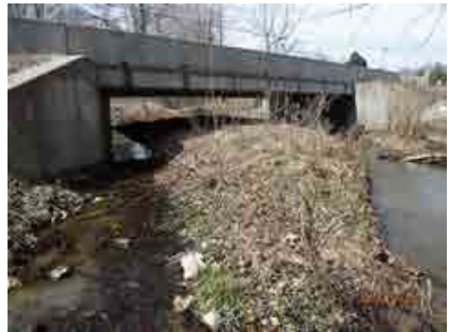
LOOKING WEST AT SILT BUILDUP
