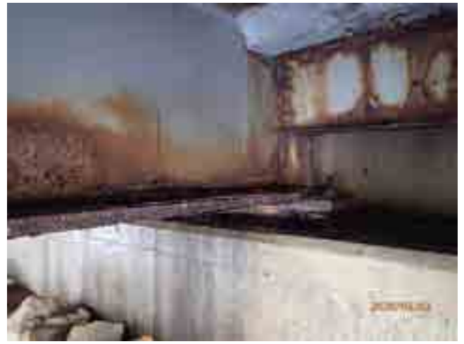
SW CORNER BEARING DETERIORATION
