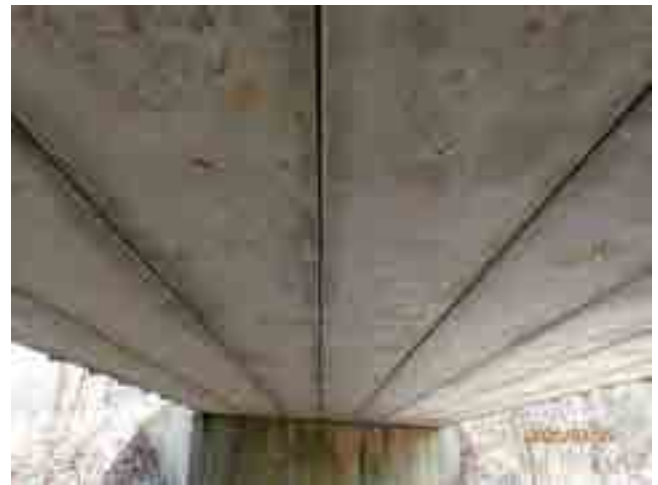
BEAM 5 AND 6 CRACKS AND DELAM.
