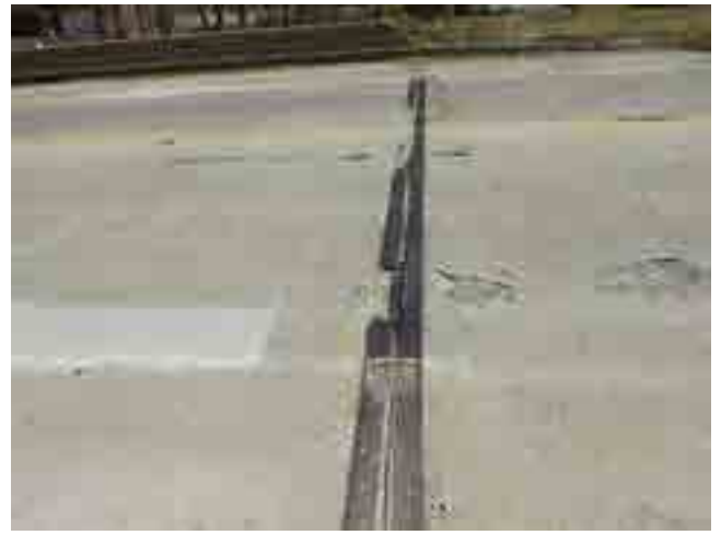
LOOKING EAST AT HEAVILY DAMAGED SOUTH JOINT
