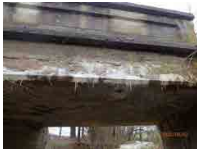
SOUTH COPING CRACKS WITH EFFL.
