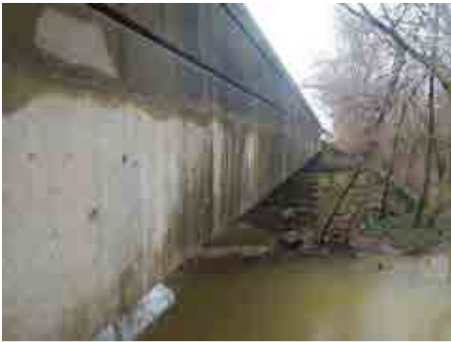
HAIRLINE CRACKS 8" ABOVE BIT. OF THE E COPING BM
