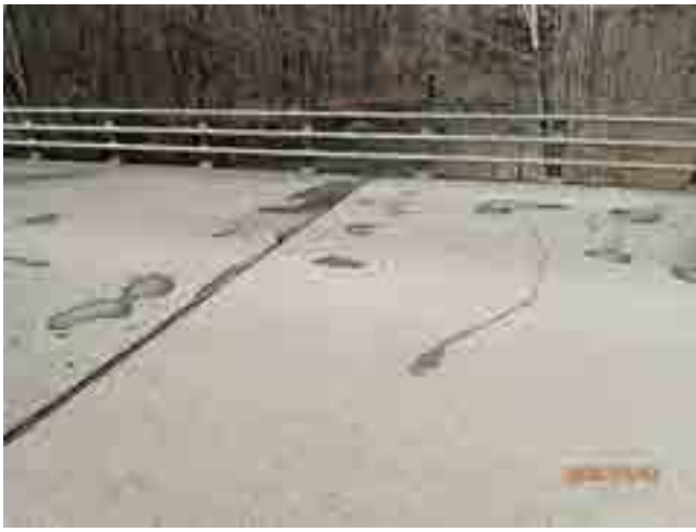
DECK SPALLS AT NORTH PIER
