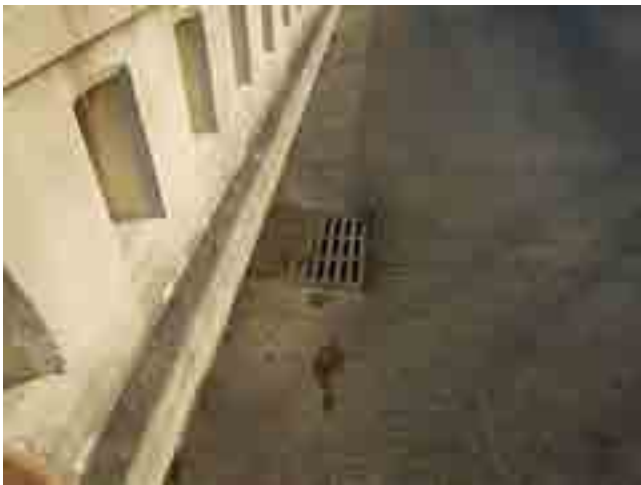
BLOCKED DECK DRAINS
