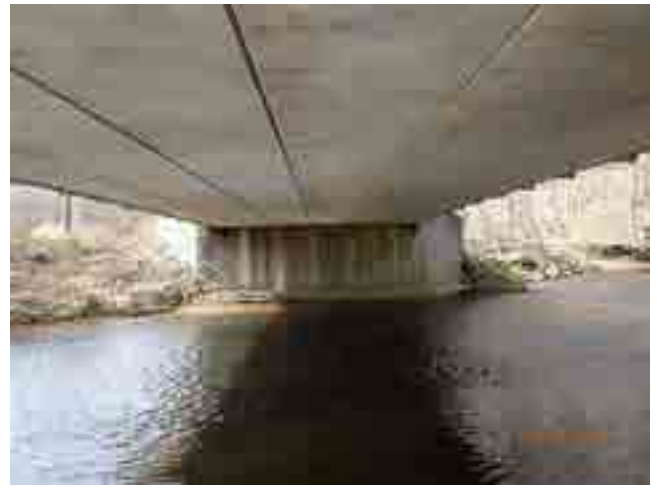
WEST ABUTMENT SCOUR
