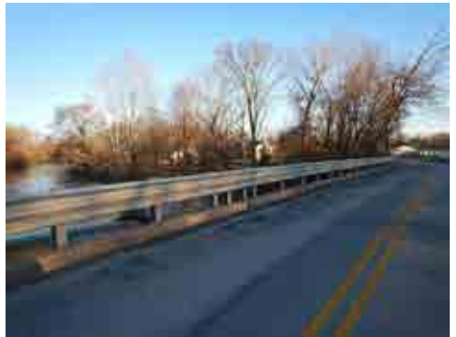
SOUTH AT PATCHED, DET. SURFACE AT PIER JOINT
