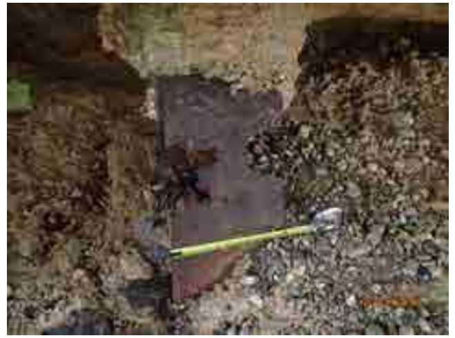
EAST ABUTMENT PILE SELECTION LOSS
