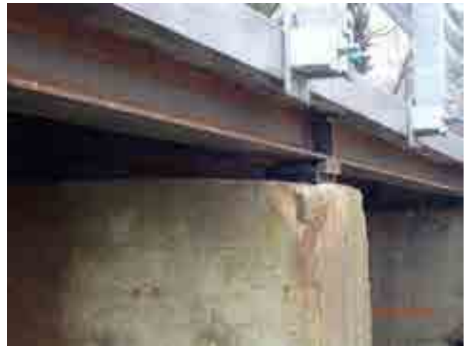
NORTH PIER BEARING SPALL
