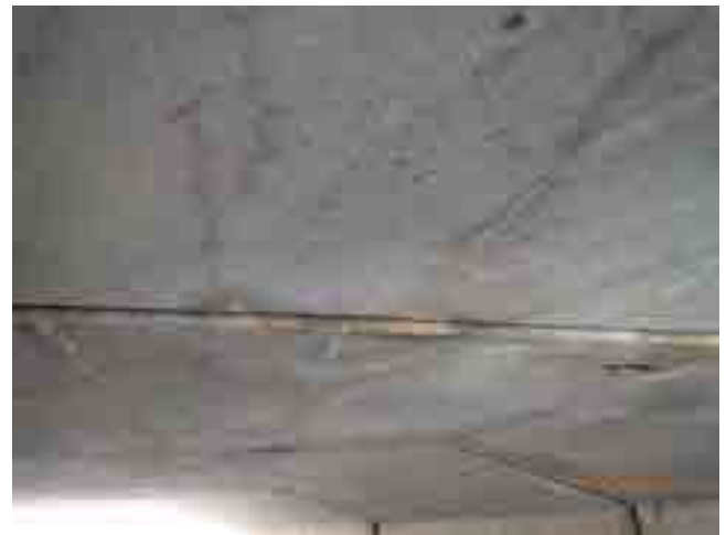
TYPICAL HAIRLINE CRACKS
