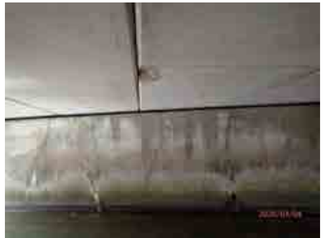
BEAM 4 SPALL NEAR WEST ABUTMENT
