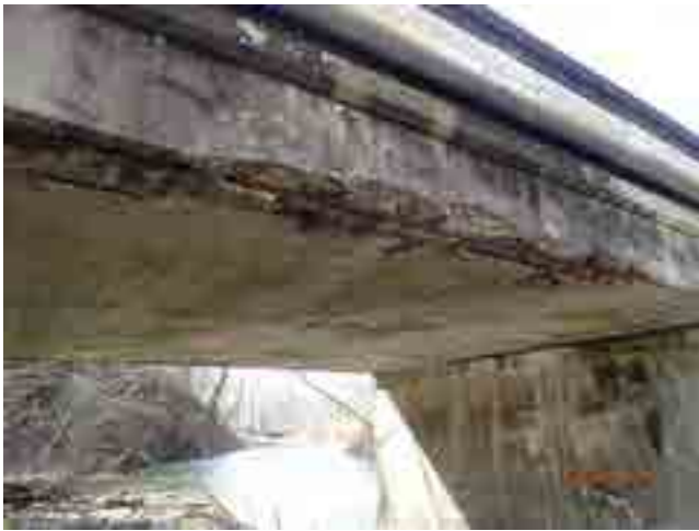
UPSTREAM, SOUTH SPAN SPALLS
