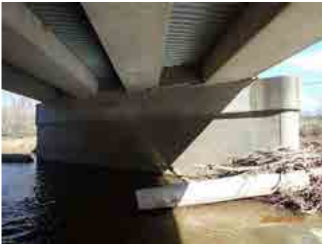
NORTH PIER WITH DEBRIS
