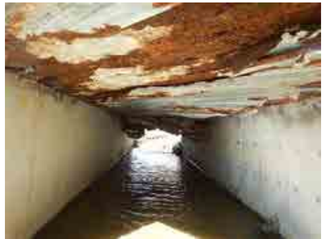
LOOKING WEST AT RUSTED CENTER SPAN METAL
