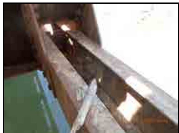
LOOKING AT L8-L10, NORTH TRUSS AT FLAKING ON OUTER CHANNEL NEAR L8
