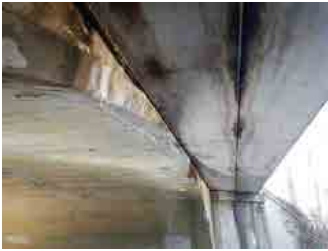
LOOKING SOUTH AT WEB ARCH COPING EFFL.
