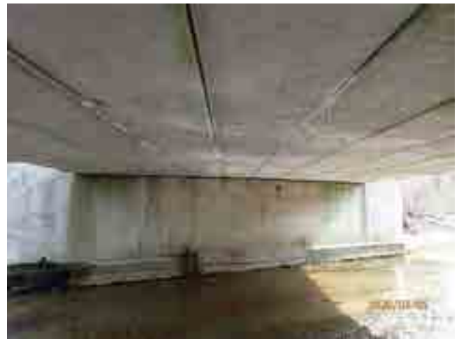
EAST ABUTMENT AND UNDERSIDE EFFL.
