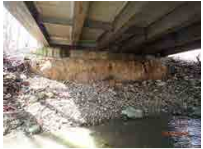
SOUTH ABUTMENT SCOUR
