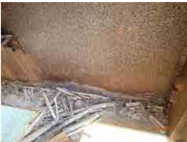
FL BEAM 4 AT FLAKING RUST NEAR S TRUSS
