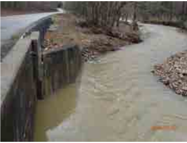
SOUTHWEST WINGWALL EROSION
