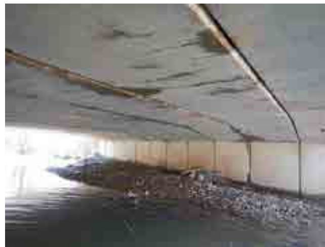
LOOKING WEST AT WATER SEEPAGE BETWEEN PRECAST
