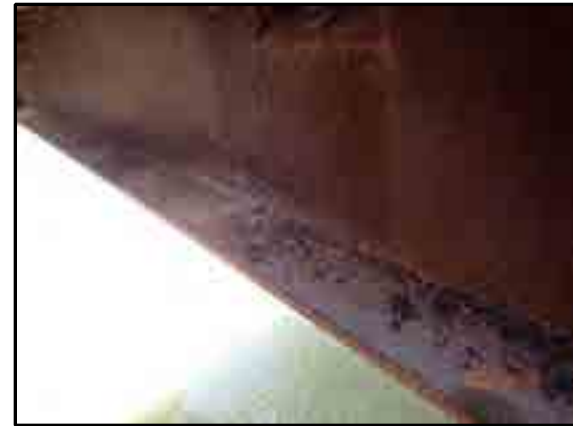
LOOKING AT FLOORBEAM 10 AT FLAKING RUST ON EAST SIDE 2.5' FROM L10, NORTH TRUSS.
