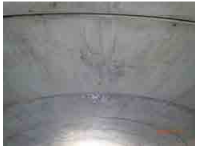
HAIRLINE CRACKS ALONG CENTERLINE
