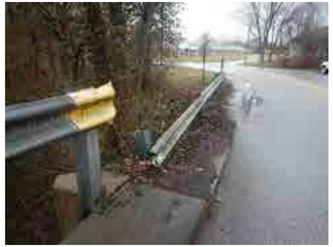
LOOKING NORTH AT DAMAGED NW APPROACH
