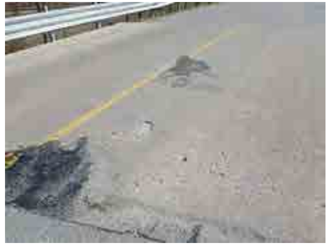
SPALLS, PATCHES, MAP CRACKING ON DECK SURFACE
