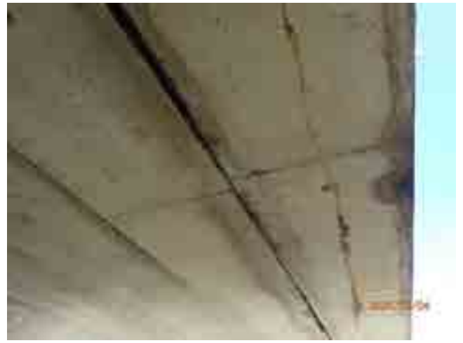
EAST BEAM CRACKS
