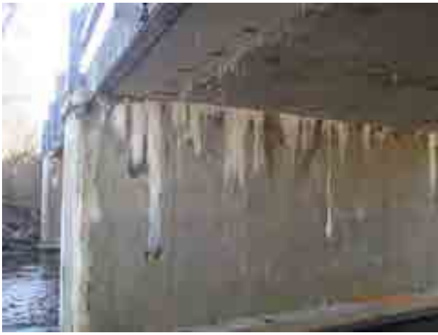
WEST PIER CAP RAVELING
