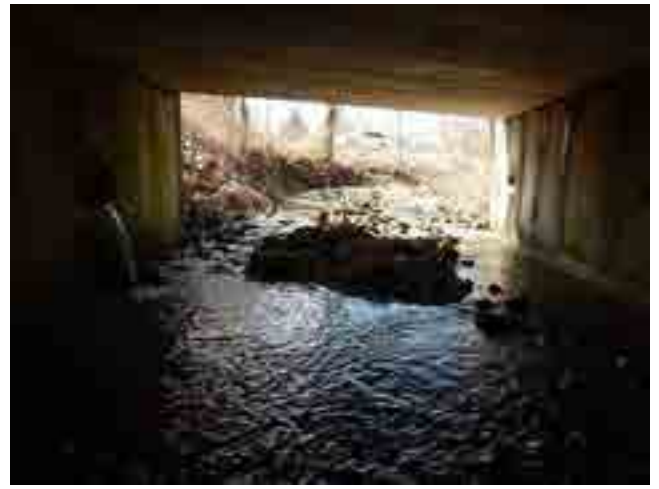
WEST AT RIPRAP MOUNDED IN CHANNEL
