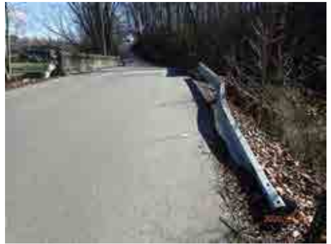
NORTHWEST GUARDRAIL DAMAGE
