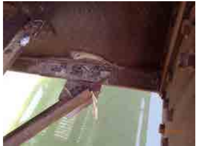
FL. BM 8, RUST ON BOTH SIDES 1" FROM L8, N TRUSS
