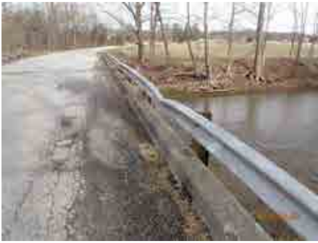
UPSTREAM GUARDRAIL DAMAGE
