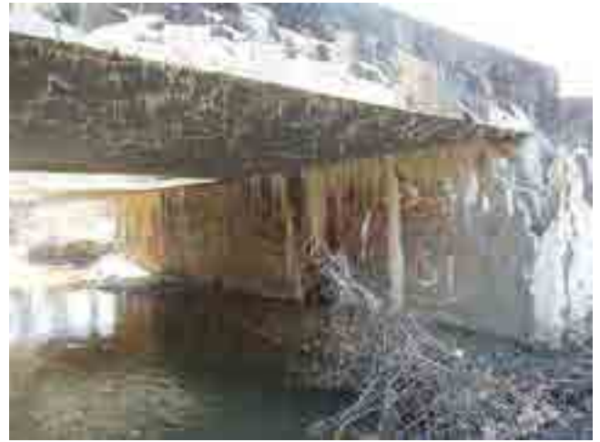
NW AT HEAVY EFFL. ON SLAB AND NORTH ABUT.
