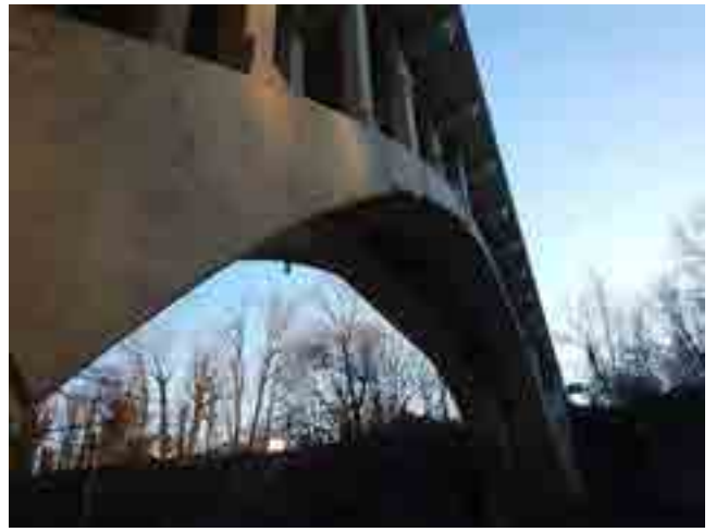
LOOKING E AT SPALLS, EXP. RESTEEL ON S COPING
