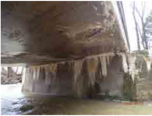
UPSTREAM EAST SPAN AND SPALLS
