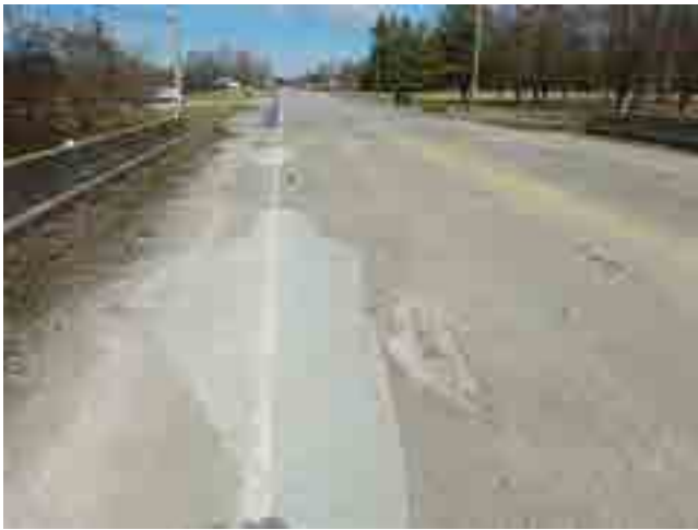
N SPALLS, PATCHES, AND HEAVY WEAR ON SURFACE
