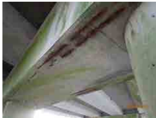
LOOKING EAST AT PIER SPALLS
