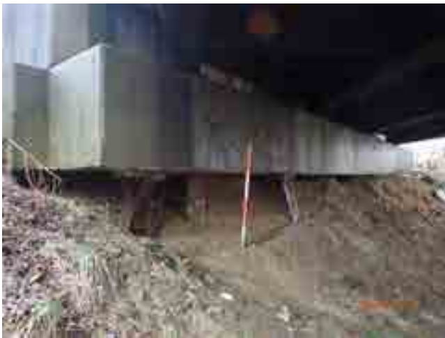
WEST ABUTMENT SCOUR
