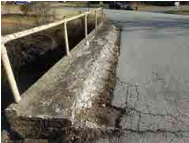
S AT HEAVY DETERIORATION OF CONCRETE AND BIT.
