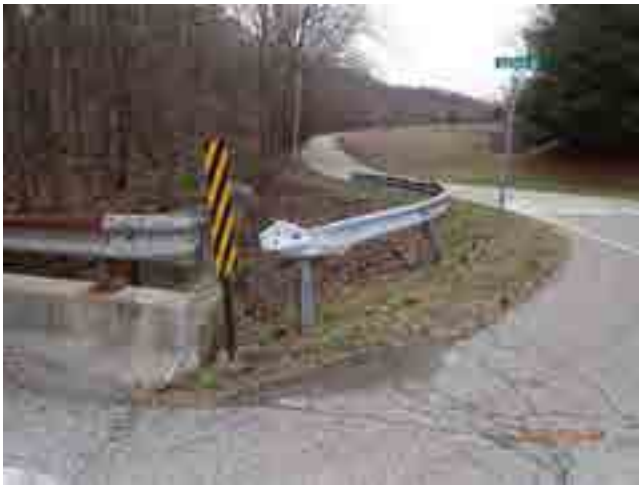
DAMAGED NW GUARDRAIL
