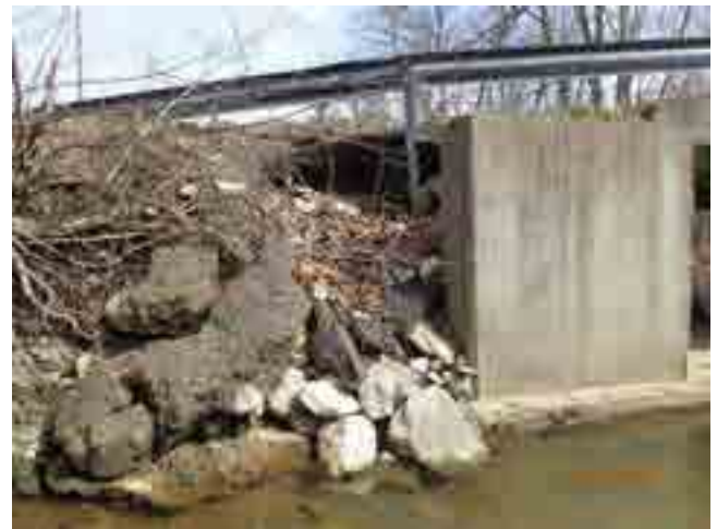
LOOKING NW AT SHOULDER EROSION
