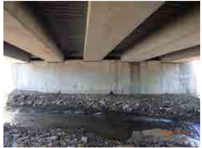
WEST ABUTMENT VERTICAL CRACKS
