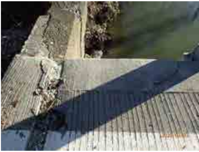
SOUTHEAST CORNER CRACK
