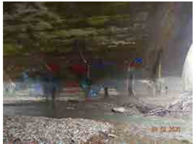
LOOKING WEST AT CRACKING, EFFL. ON WEST ABUT.,
