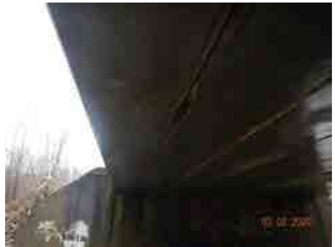
LOOKING SOUTH AT CRACK IN BEAM 9 AT EAST COPING
