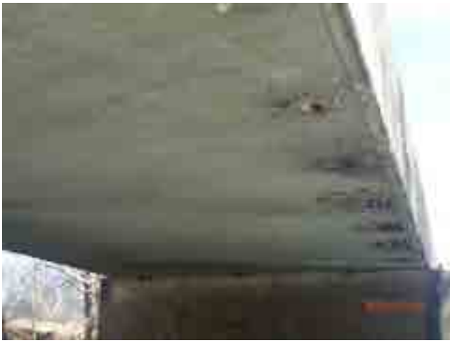
CENTER SPAN SPALLS
