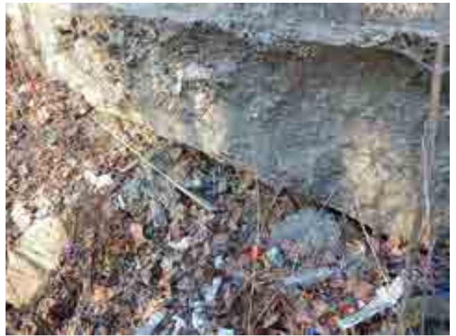
EAST AT UNDERMINED SW CORNER OF APPR.
