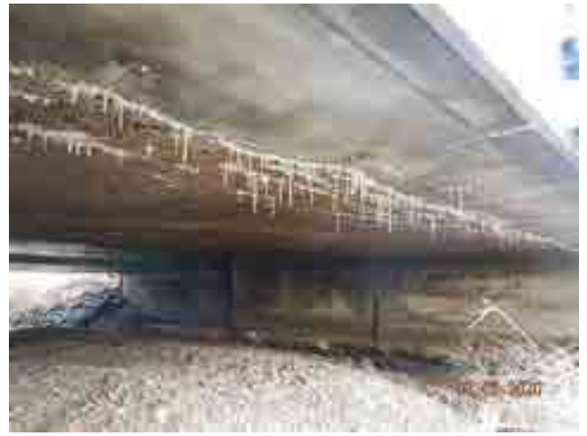
LOOKING SOUTH AT EFFL. IN SOUTH SPAN SLAB
