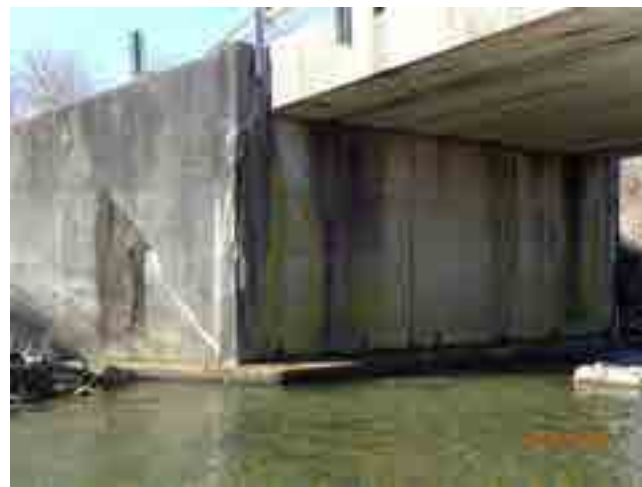
SOUTHEAST CORNER CRACKS
