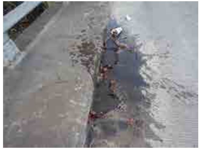
SPALLS IN W GUTTER LINE, WITH EXP. RESTEEL
