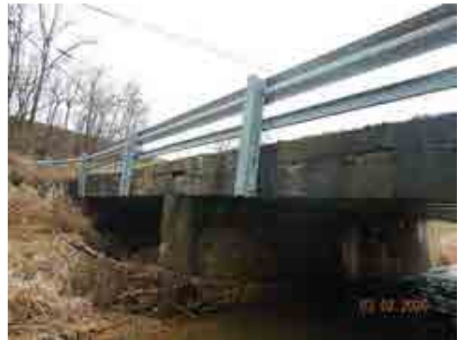
LOOKING SOUTH CRACKED, SPALLING EAST COPING
