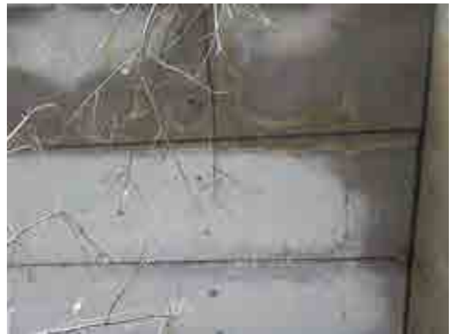
HAIRLINE CRACK IN BOTTOM BEAM 10 AT EAST COPING
