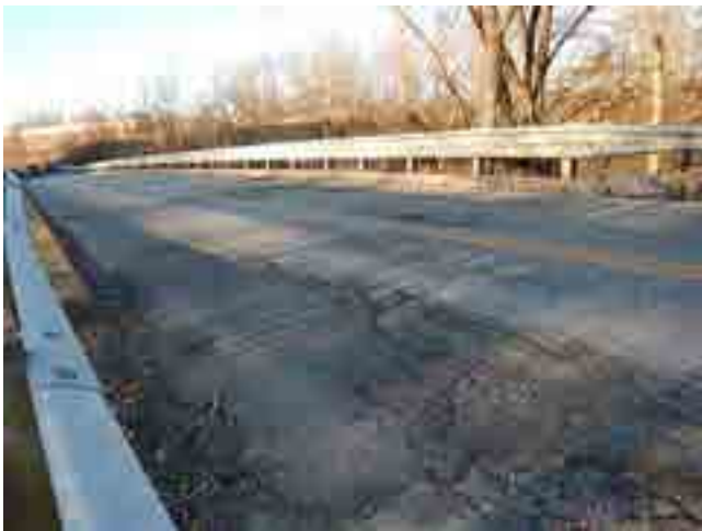
NORTH AT DET. AND SETTLING SOUTH ROADWAY APPR.
