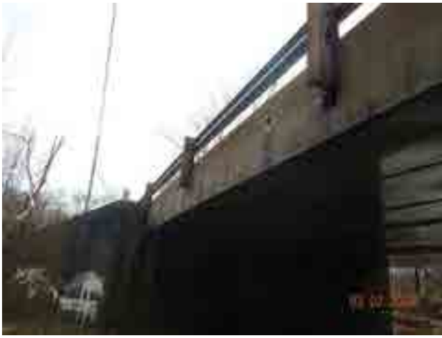
LOOKING SOUTH AT CRACK IN SIDE OF BEAM 9 WITH
