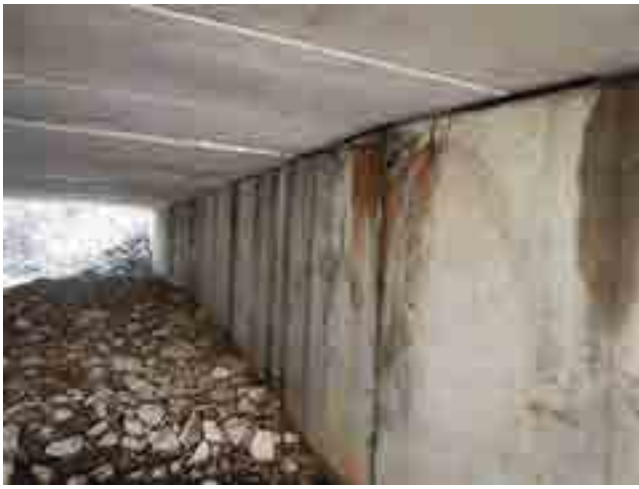
S HAIRLINE CRACKS, EFFL. RUST STAINS ON W ABT.
