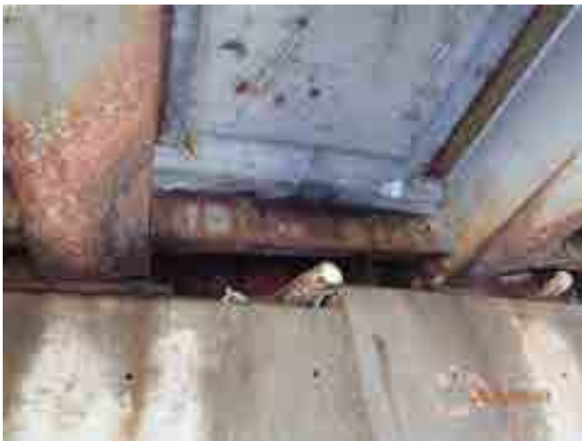
NORTH PIER BEARING DETERIORATION
