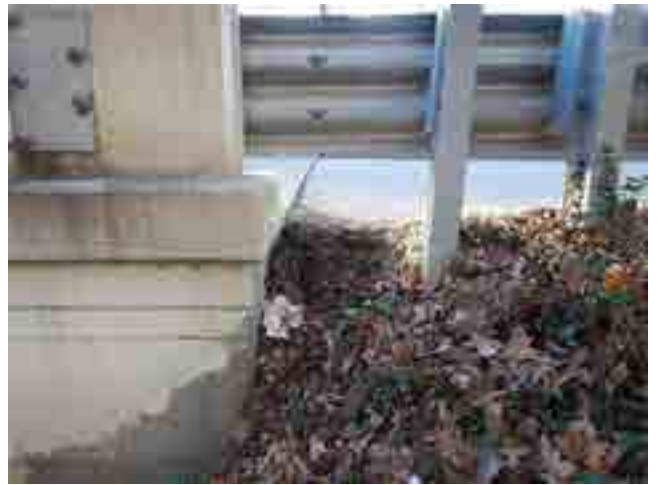
LOOKING SOUTH AT EROSION AT NORTHWEST BRIDGE
