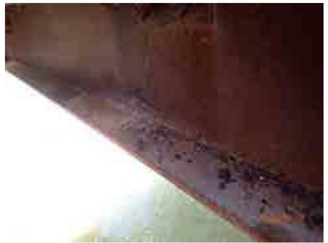
FL BM 10, FLAKING RUST ON E SIDE 2.5' FROM L10, N
