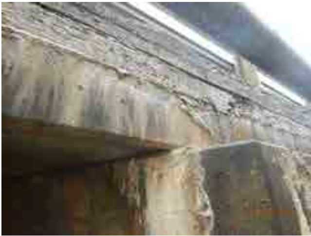
SOUTH BOX BM DETERIORATION OVER THE PIER
