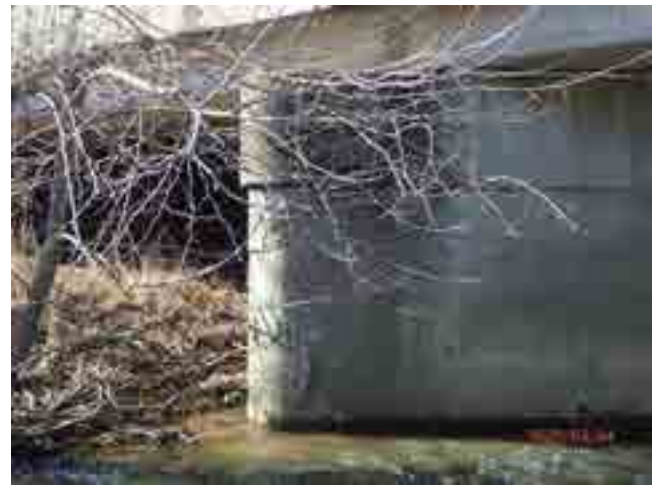
SPALLS AT UPSTREAM OF SOUTH PIER
