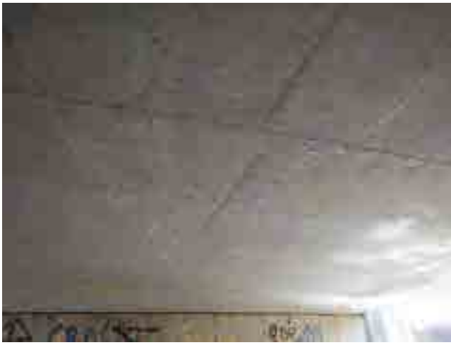
S HAIRLINE CRACKS WITH EFFL. ON BTM. OF SLAB
