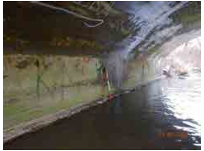
LOOKING SOUTH AT SCOUR ALONG THE EAST ABUT.
