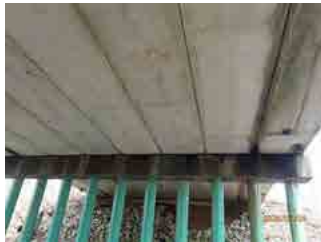
NORTH PIER BEAM END CRACKS
