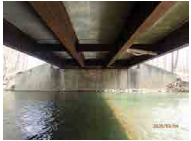
EAST ABUTMENT SCOUR
