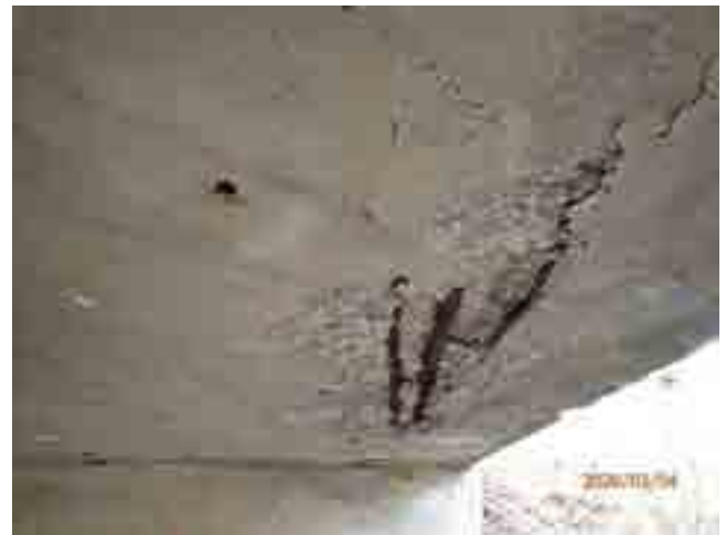
LOOKING NORTH SPAN SPALL
