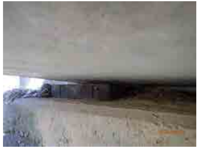
NE BRIDGE WITH OUT BEAM CONTACT
