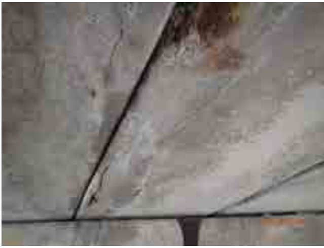
BEAM 6 CRACK WITH RUST STRAINS
