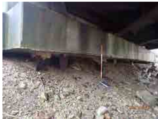
LOOKING EAST AT ABUTMENT SCOUR
