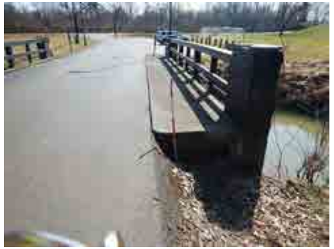
LOOKING EAST AT SW CORNER DROP OFF AT PAVEMENT
