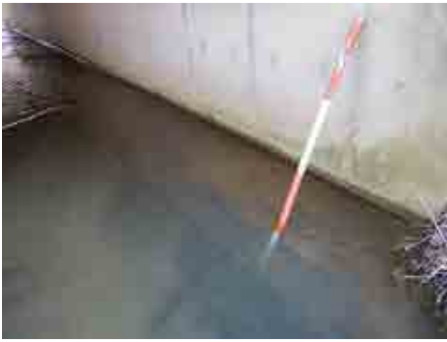
LOOKING SOUTHEAST AT EXPOSED FOOTING ON PIER
