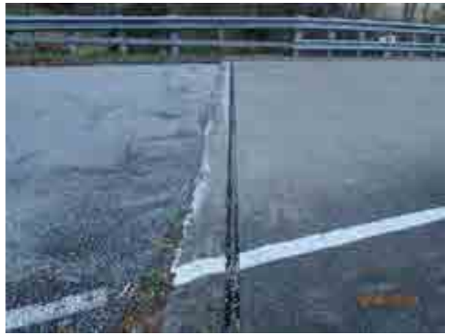
WEST BRIDGE END DAMAGE
