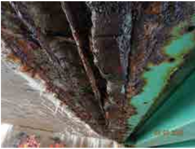
LOOKING NORTH AT SPALLED SLAB, EXPOSED RESTEEL,
