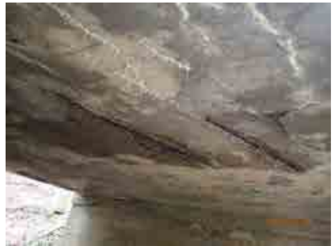
NORTH SPAN SPALLS
