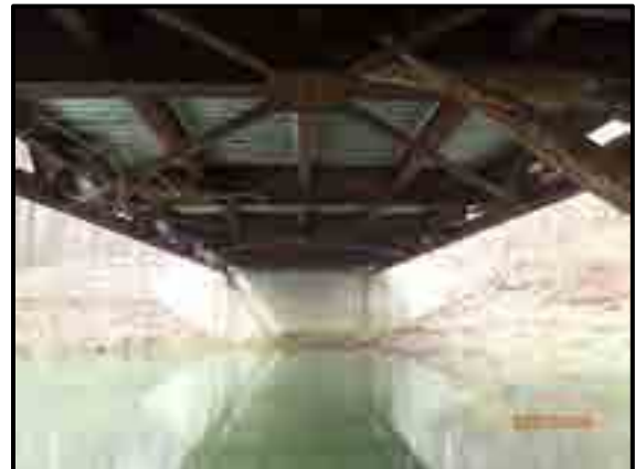
LOOKING WEST AT UNDERSIDE DEBRIS
