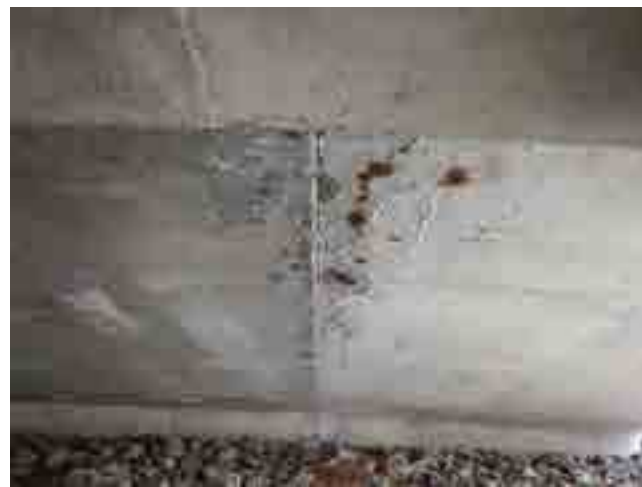
LOOKING SOUTH AT SPAN CRACKING WITH EFFL.
