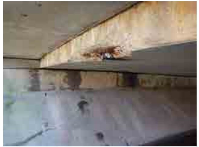
LOOKING AT SPALL WITH EXPOSED BROKEN STRANDS
