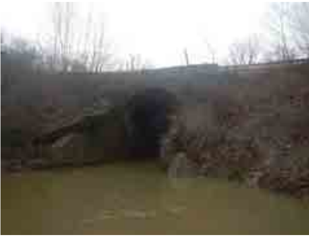
NW AT BROKEN HEADWALLS, GABIONS ABOVE
