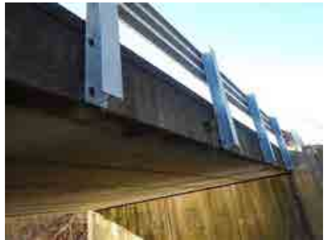
HAIRLINE CRACK IN NORTH COPING BEAM AT
