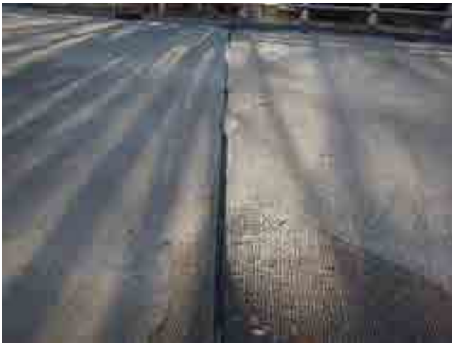
LOOKING WEST AT DAMAGED JOINT MATERIAL
