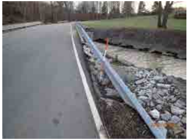
NORTHEAST SHOULDER EROSION
