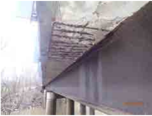
NW COPING SPALLS, LOOKING EAST
