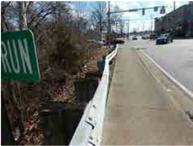
LOOKING SOUTH AT DAMAGED SOUTH APPROACH
