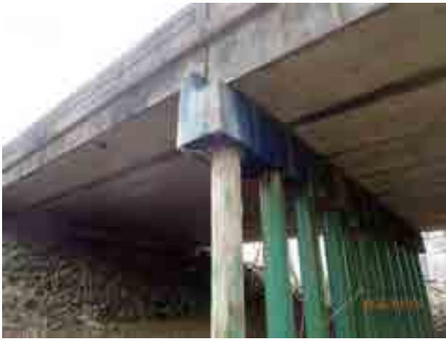
SOUTHEAST PIER BEAM END CRACKS
