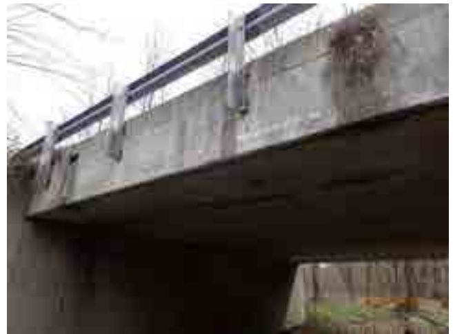
DOWNSTREAM BEAM CRACKS AND EFFL.
