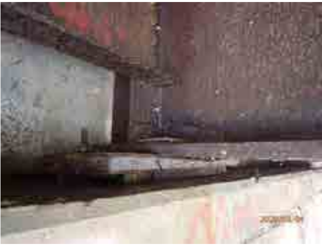
WEST ABUTMENT BEAM 2 BEARING DETERIORATION
