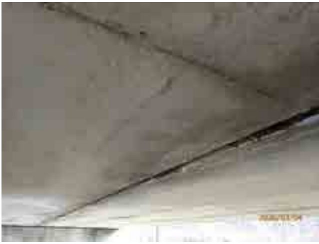
BEAM 3 HAIRLINE CRACK
