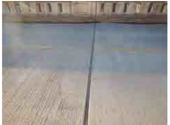
LOOKING AT DIRT FILLED BRIDGE JOINT
