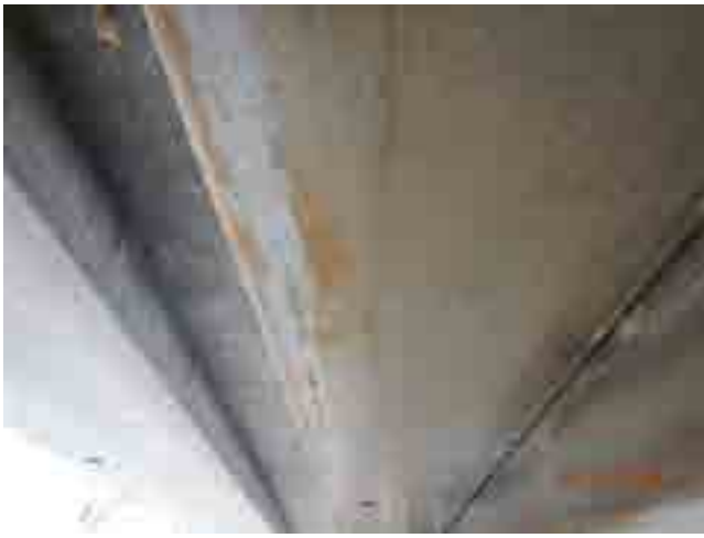
LOOKING WEST AT SEALED CRACK IN BEAM 6
