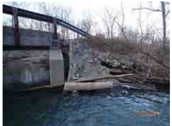
SOUTHEAST CORNER SCOUR
