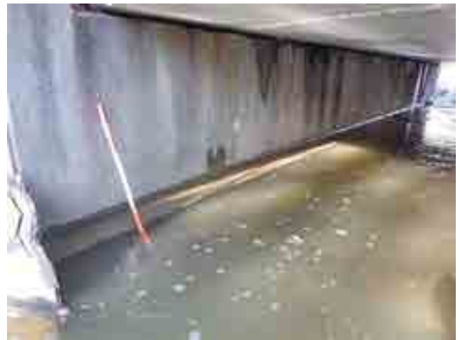
LOOKING EAST AT SCOUR ALONG THE NORTH
