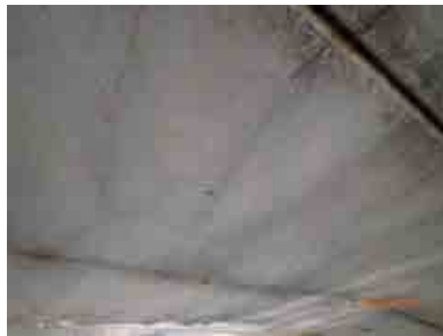
TYPICAL HAIRLINE CRACK
