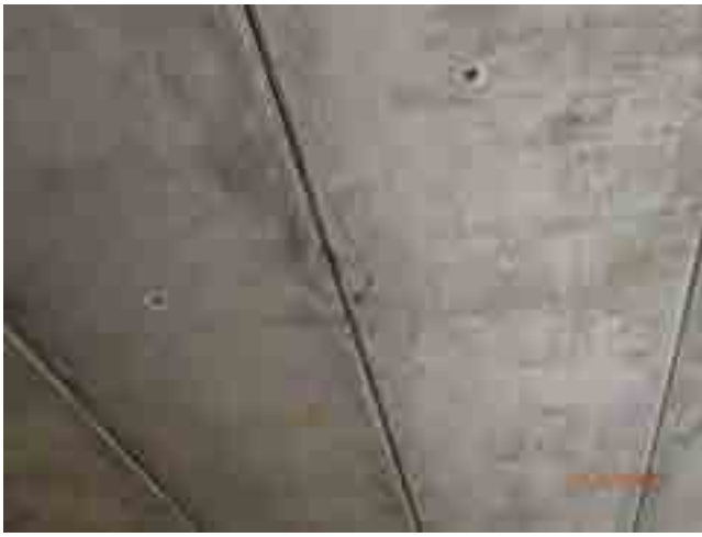
BEAM 3 CRACK AND DELAM.
