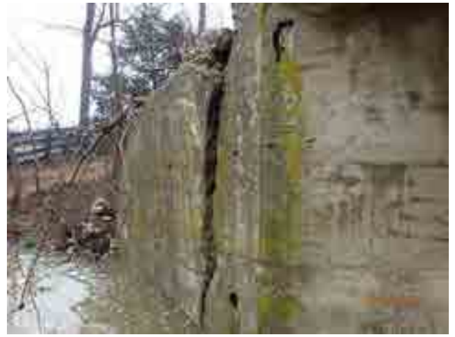
NORTHEAST WINGWALL FAILURE
