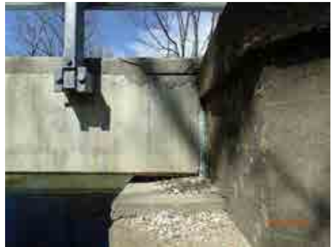
SE BEAM WITH DECK CRACKS
