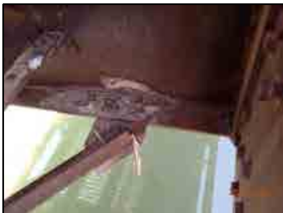
LOOKING AT FLOORBEAM 8 AT FLAKING RUST ON BOTH SIDES 1' FROM L8, NORTH TRUSS.
