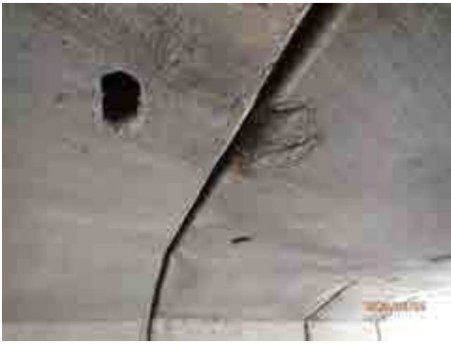
SPALL AT MIDSPAN
