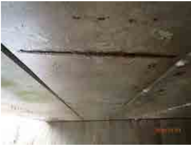
BEAM 3 EXPOSED STRAP
