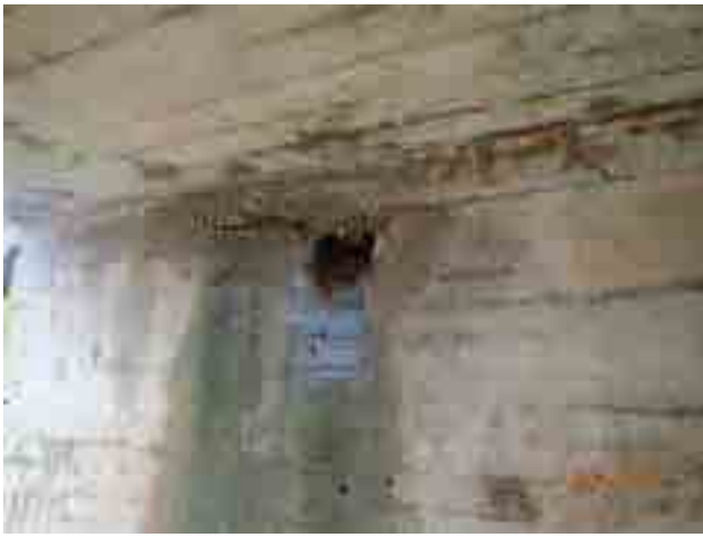
EAST ABUTMENT SPALL
