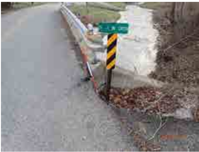
LOOKING NORTHWEST CORNER EROSION
