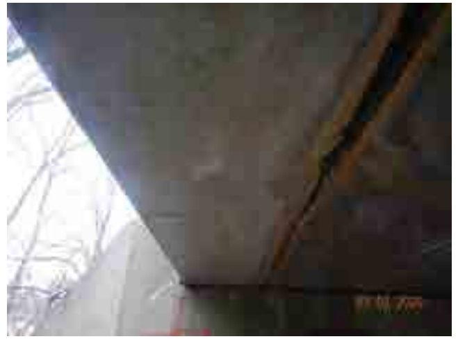
LOOKING NORTH AT HAIRLINE CRACKS IN BEAM 1
