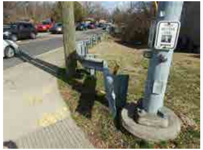
EAST AT DAMAGED SOUTHWEST APPROACH RAILING
