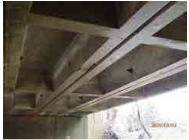
UPSTREAM SPALL AND WEB CRACKS
