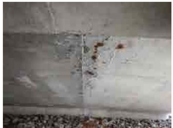
LOOKING SOUTH AT SPAN CRACKING WITH EFFL.
