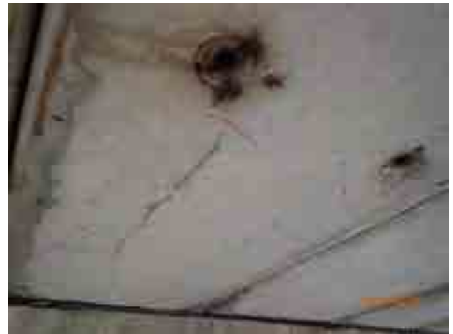
TYPICAL HAIRLINE CRACKS AT BEAM ENDS
