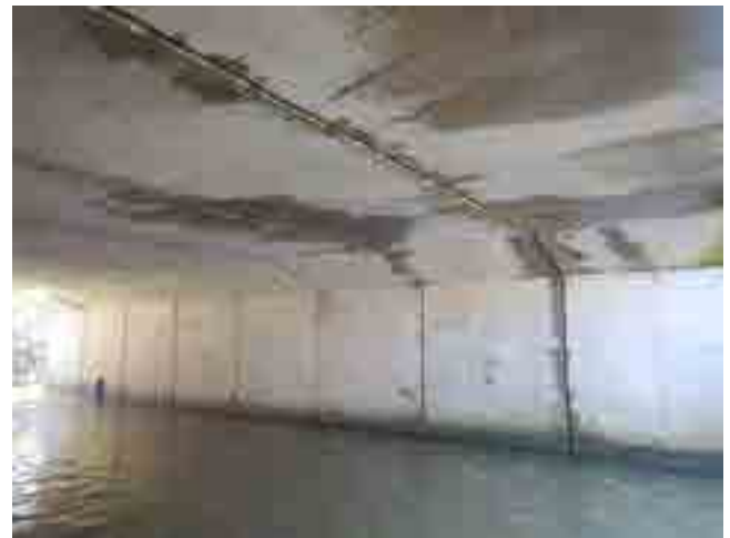
LOOKING WEST AT WATER SEEPAGE, EFFL AT JOINTS
