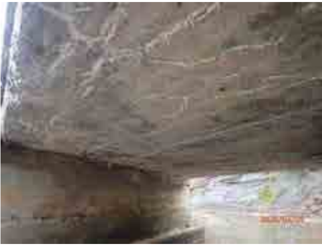
SOUTH SPAN CRACKS WITH EFFL.
