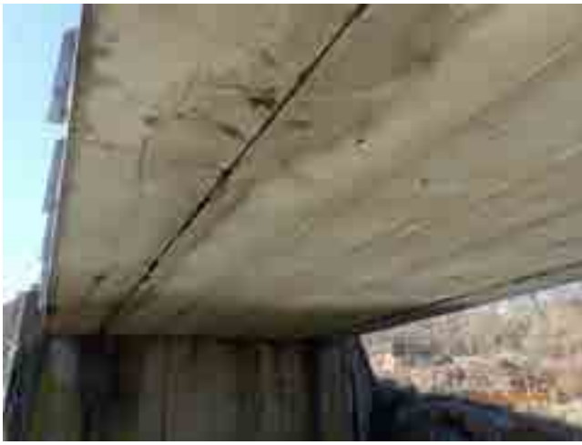
SOUTH UNDERSIDE CRACKS
