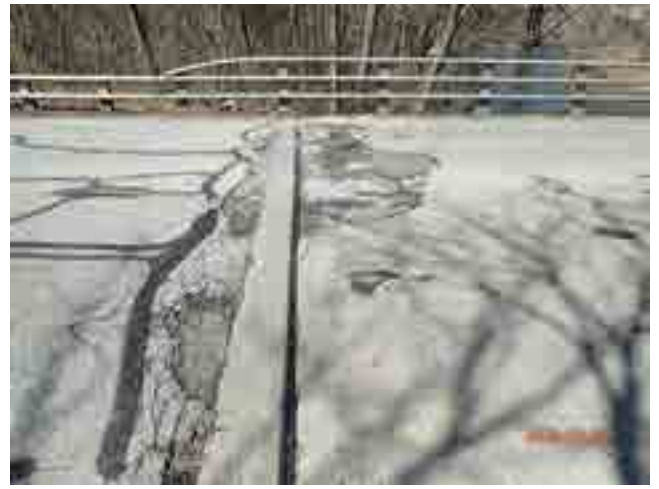
DECK SPALLS AT SOUTH ABUTMENT
