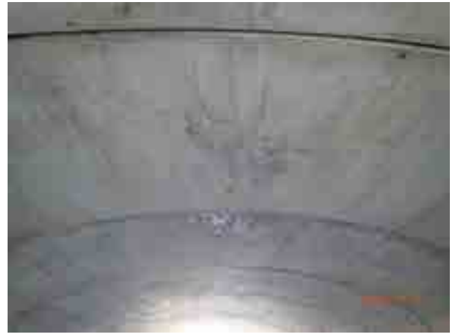
HAIRLINE CRACKS ALONG CENTERLINE
