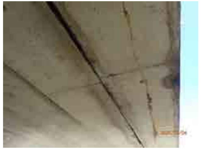
EAST BEAM CRACKS
