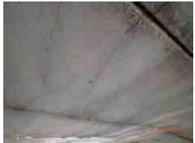
TYPICAL HAIRLINE CRACK
