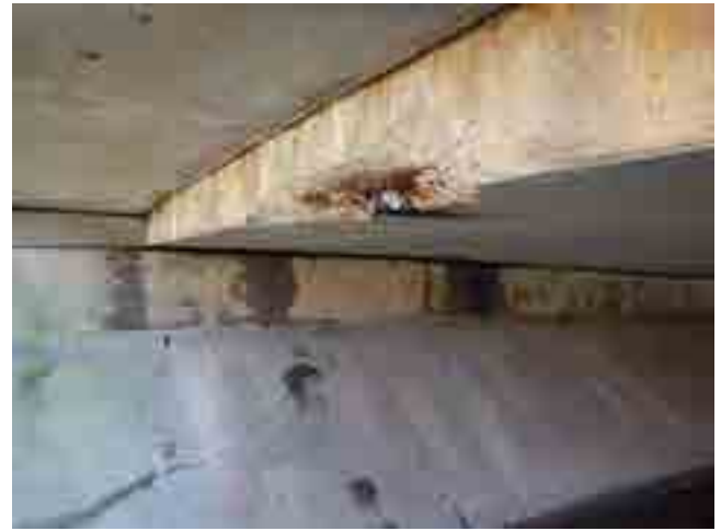
LOOKING AT SPALL WITH EXPOSED BROKEN STRANDS
