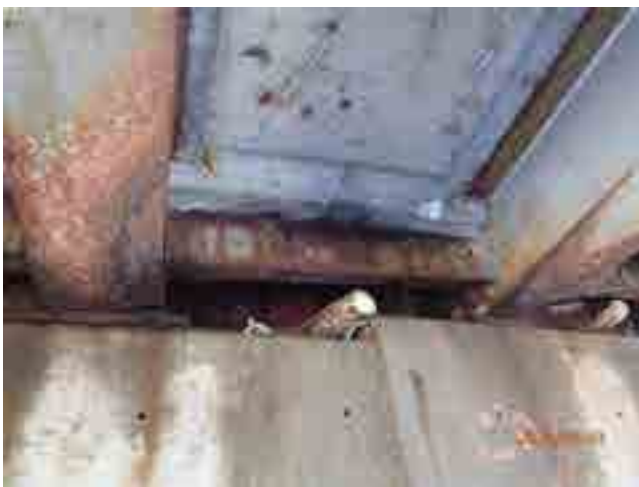
NORTH PIER BEARING DETERIORATION
