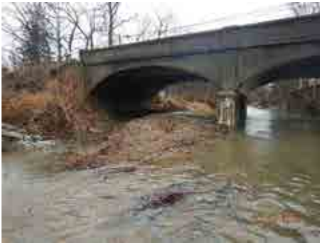
LOOKING NORTH AT AGGREGATION IN WEST SPAN
