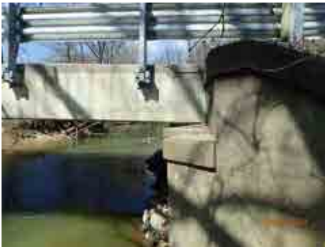
SE BEAM WITH DECK CRACKS
