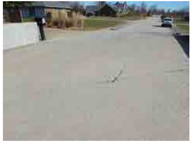
LOOKING NORTH AT LONGITUDINAL CRACK IN PIER
