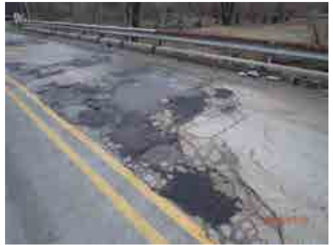
WEST END DECK SPALLS/ PATCHES
