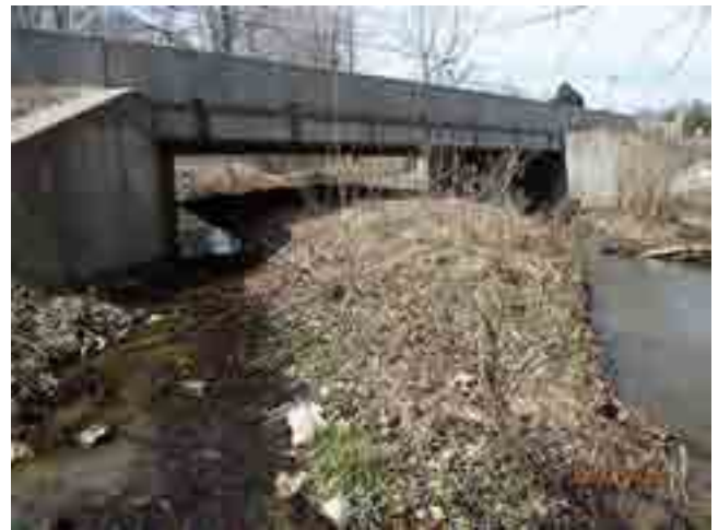
LOOKING WEST AT SILT BUILDUP
