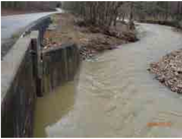
SOUTHWEST WINGWALL EROSION
