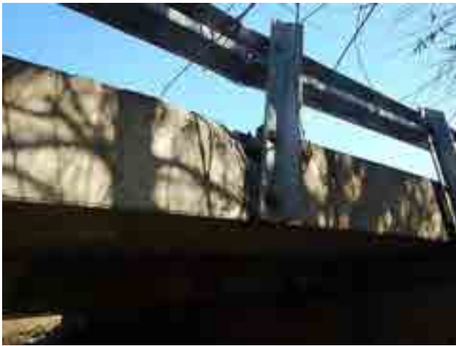
LOOKING SOUTH COPING SPALL AT POST CONNECTION
