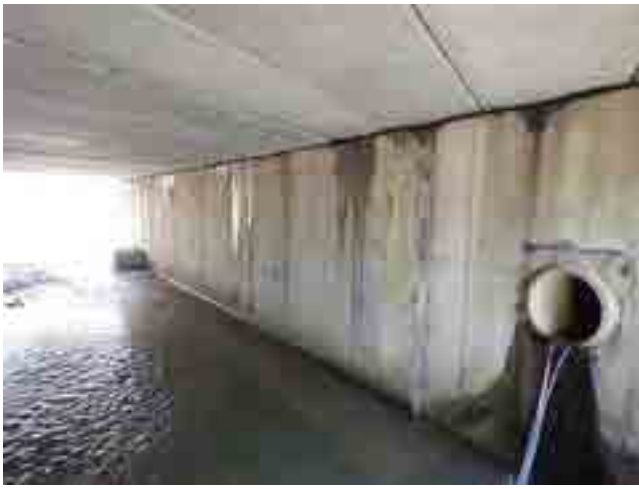
H'LINE CRACKS IN S ABT. WITH SPALLS AND DELAMS.
