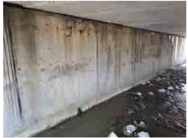
NE HAIRLINE CRACKS IN THE NORTH ABUT.
