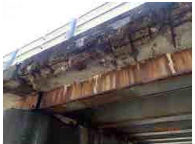
D/S COPING SPALLS AT NORTH PIER
