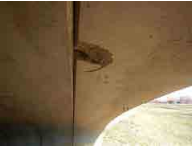
LOOKING NORTH AT SPALL ON EAST COPING PRECAST
