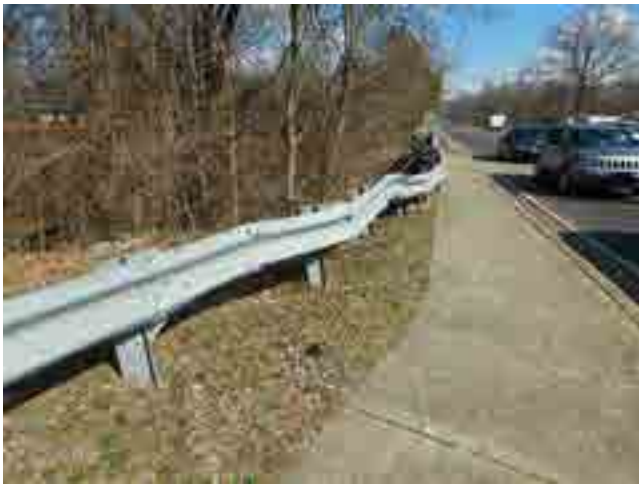
EAST AT DAMAGED NORTHWEST APPR. RAILING
