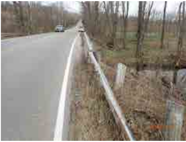
SE CORNER GUARDRAIL DAMAGE
