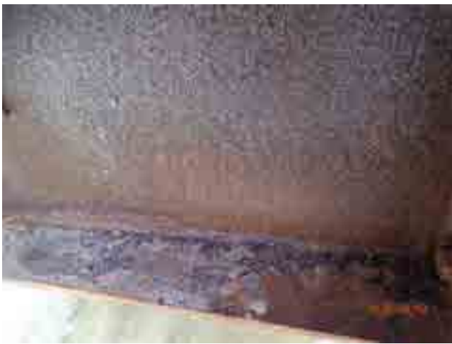
FL BM 2, FLAKING RUST ON E SIDE 1' FROM L2, N TRUSS
