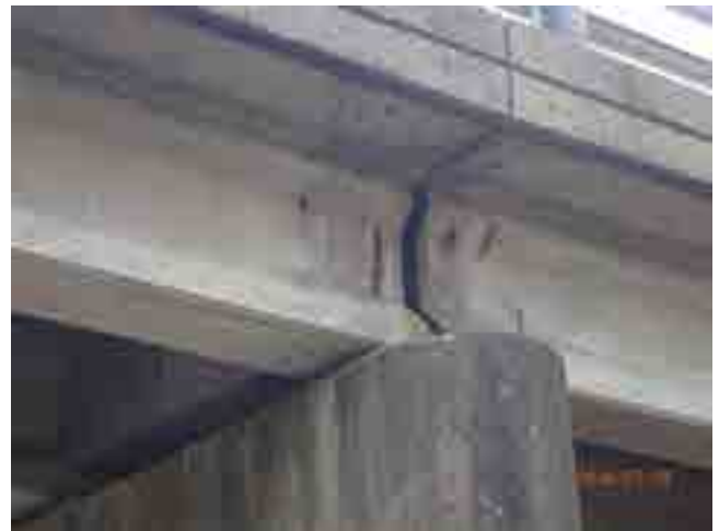
UPSTREAM N PIER BM SPALL
