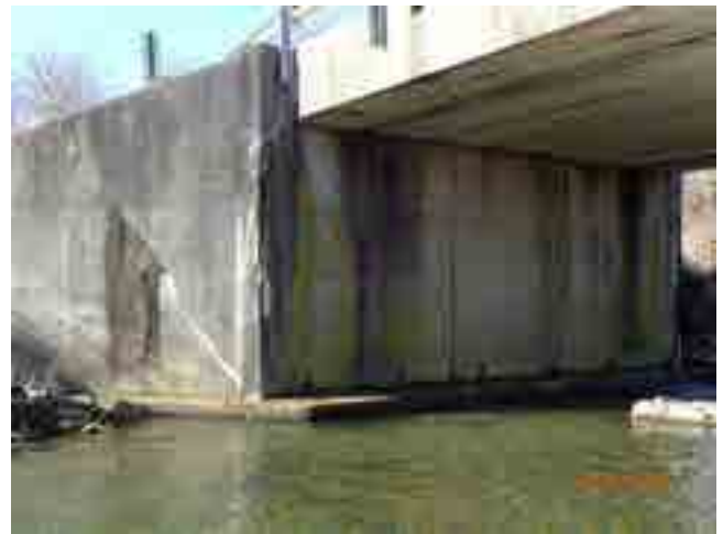
SOUTHEAST CORNER CRACKS
