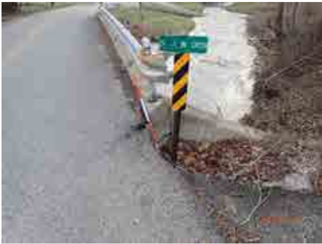
LOOKING NORTHWEST CORNER EROSION
