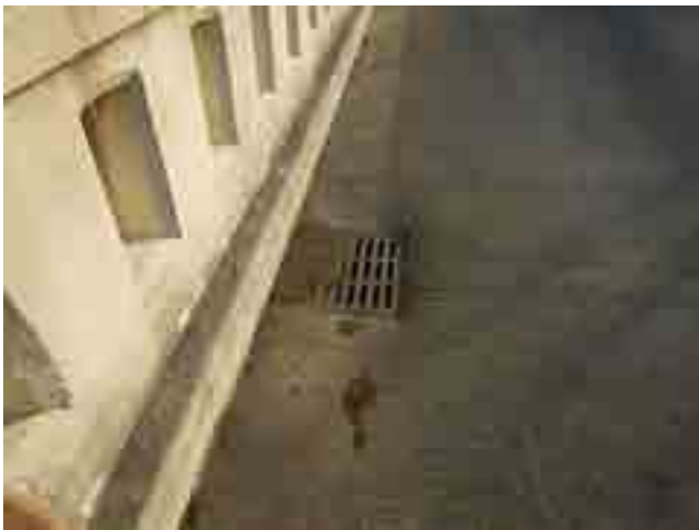
BLOCKED DECK DRAINS
