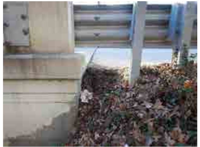
LOOKING SOUTH AT EROSION AT NORTHWEST BRIDGE
