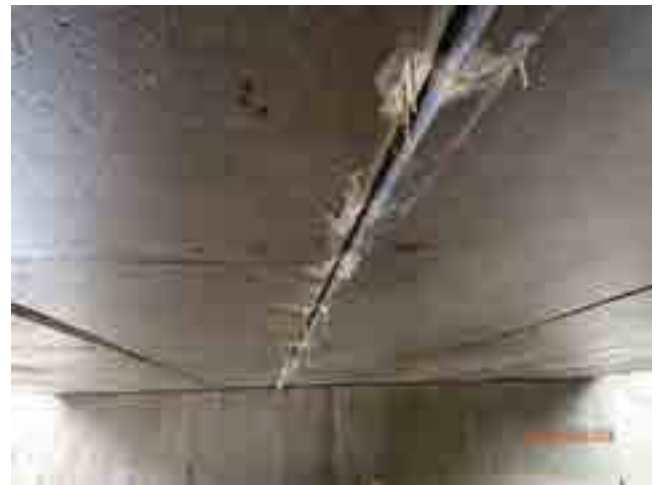
BEAM SEEPAGE NEAR CENTERLINE BRIDGE
