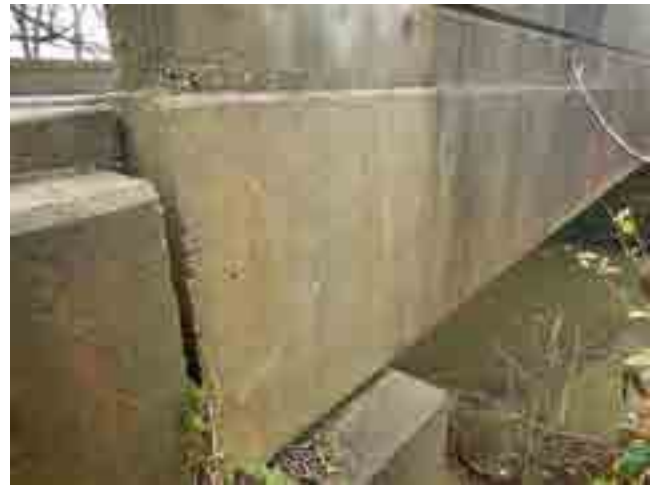
HAIRLINE CRACKS AT NORTH OF WEST COPING BEAM
