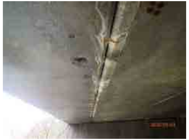
BEAM 1 SPALL AND SEEPAGE
