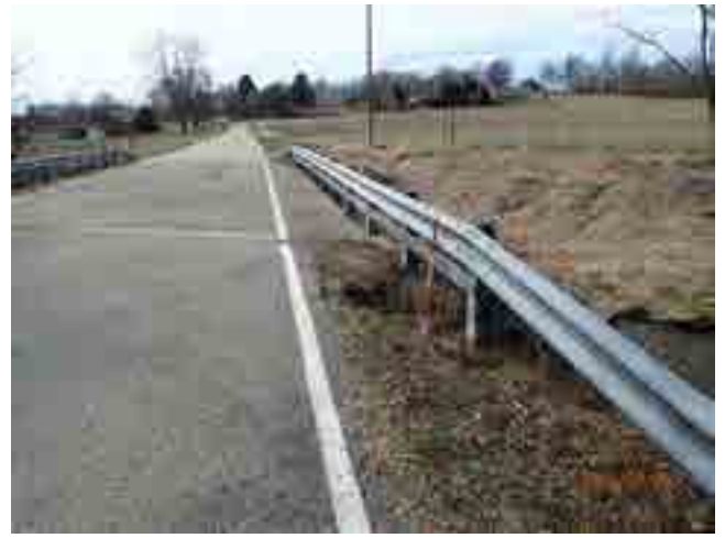
NORTHEAST SHOULDER EROSION
