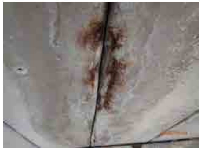
BEAMS 5 & 6 EXPOSED AND BROKEN STRANDS
