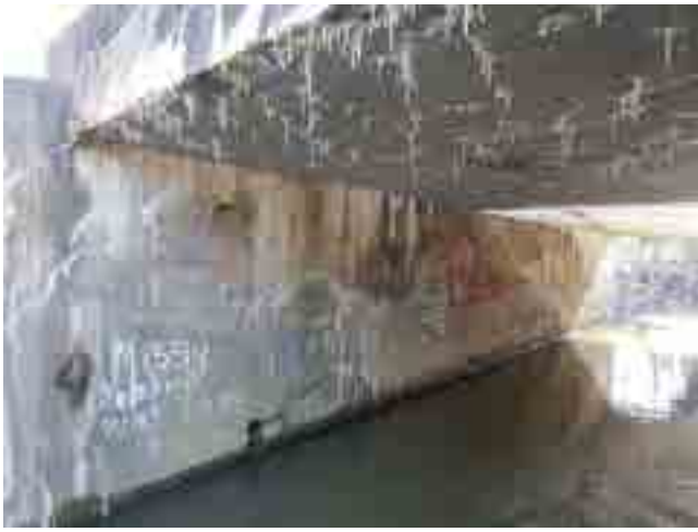
SW AT HEAVY EFFL. ON SLAB AND SOUTH ABUT.
