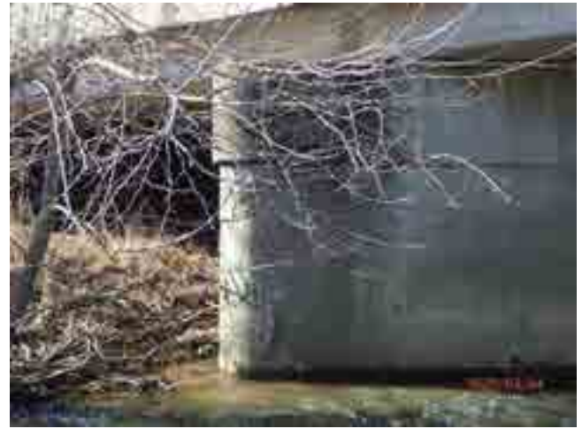
SPALLS AT UPSTREAM OF SOUTH PIER
