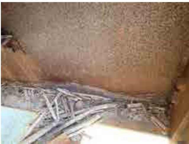
FL BEAM 4 AT FLAKING RUST NEAR S TRUSS
