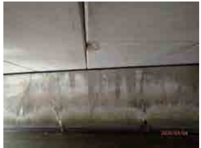
BEAM 4 SPALL NEAR WEST ABUTMENT
