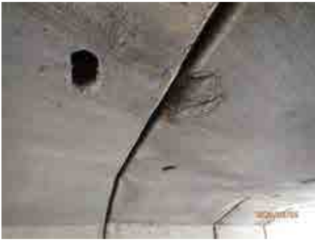
SPALL AT MIDSPAN
