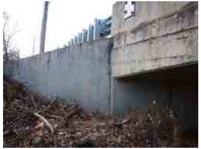
SPALL AT SOUTHWEST WINGWALL CORNER
