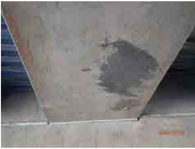
BEAM 4 GROUTED HAIRLINE CRACKS
