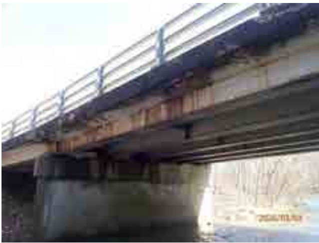
DOWNSTREAM COPING SPALLS
