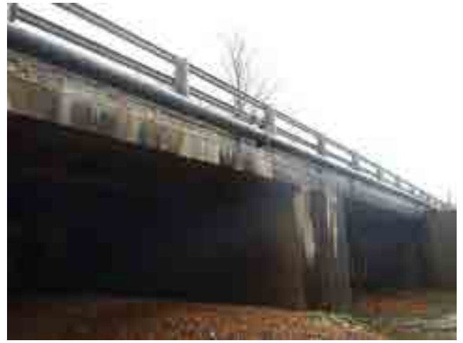
LOOKING SOUTHEAST AT HEAVY EFFL. ALONG WEST
