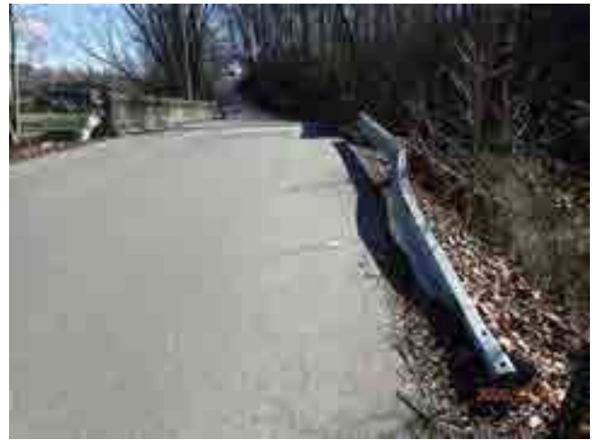
NORTHWEST GUARDRAIL DAMAGE
