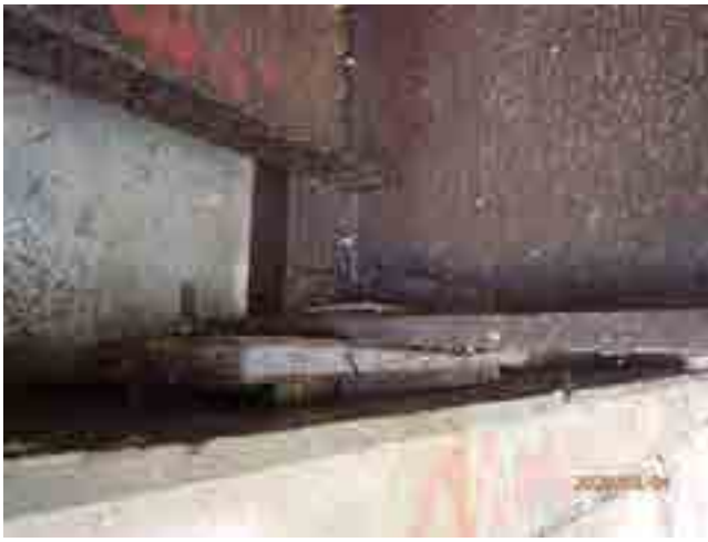
WEST ABUTMENT BEAM 2 BEARING DETERIORATION
