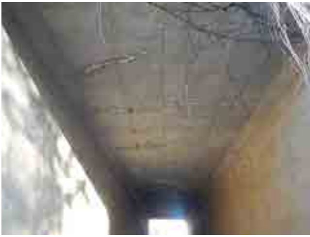
LOOKING WEST AT CRACKS IN BOTTOM OF CONCRETE
