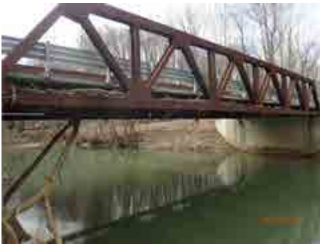
UPSTREAM DEBRIS IN LOWER CHORDS
