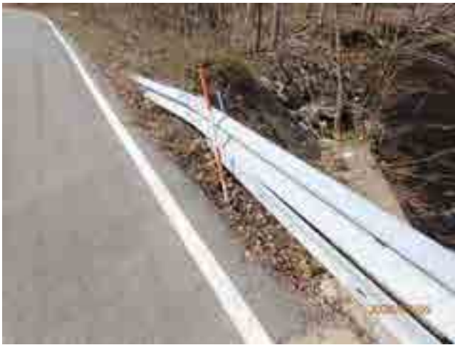
NW CORNER SHOULDER EROSION
