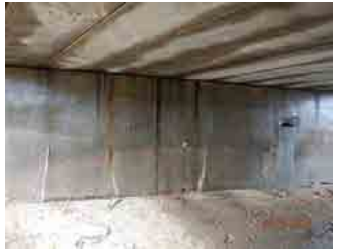
LOOKING WEST AT CRACKS IN THE WEST BENT
