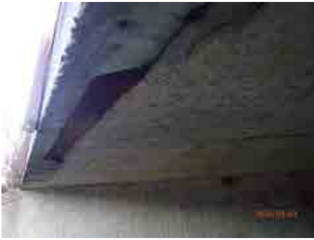
DOWNSTREAM COPING SPALL
