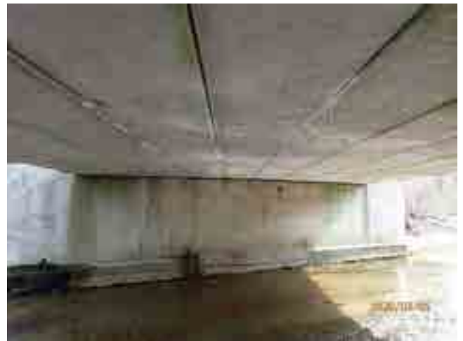
EAST ABUTMENT AND UNDERSIDE EFFL.
