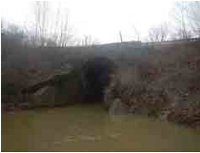
NW AT BROKEN HEADWALLS, GABIONS ABOVE
