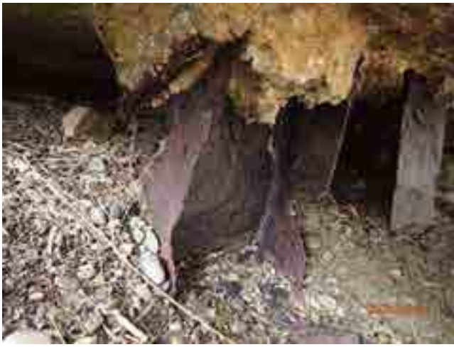
NE ABUTMENT PILE SELECTION LOSS
