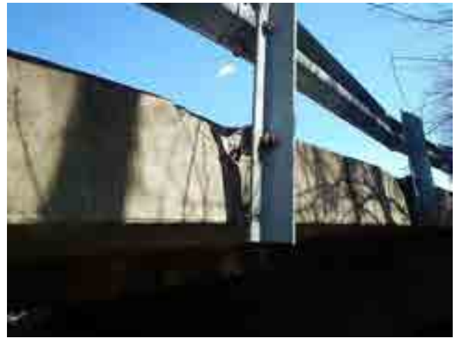
LOOKING SOUTH AT COPING SPALL AT POST
