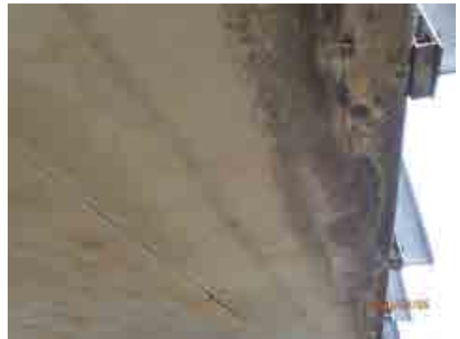
SOUTH COPING BEAM CRACK
