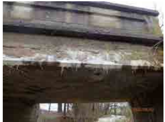
SOUTH COPING CRACKS WITH EFFL.
