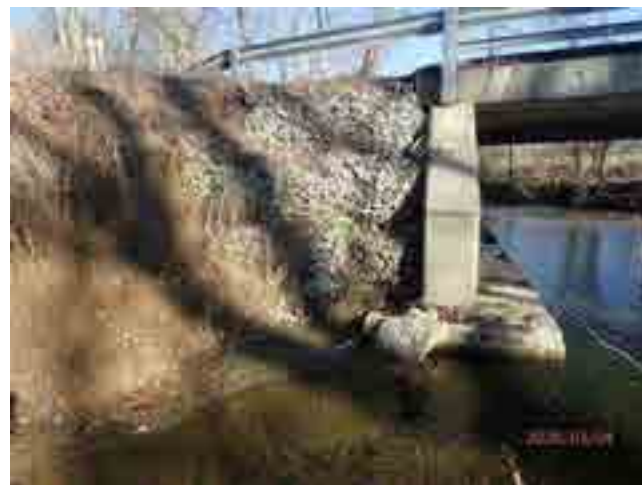
SOUTHWEST CORNER SCOUR
