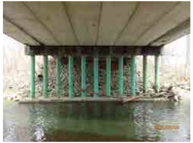
NORTH PIER SCOUR
