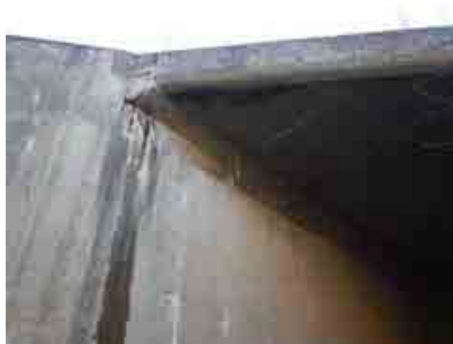
LOOKING EAST AT HAIRLINE CRACKS WITH EFFL. AT THE
