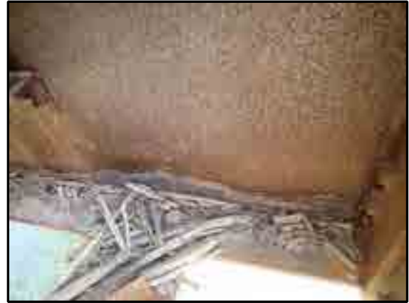
LOOKING AT FLOORBEAM 4 AT FLAKING RUST NEAR SOUTH TRUSS.
