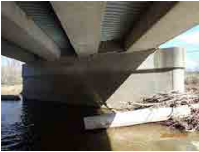
NORTH PIER WITH DEBRIS
