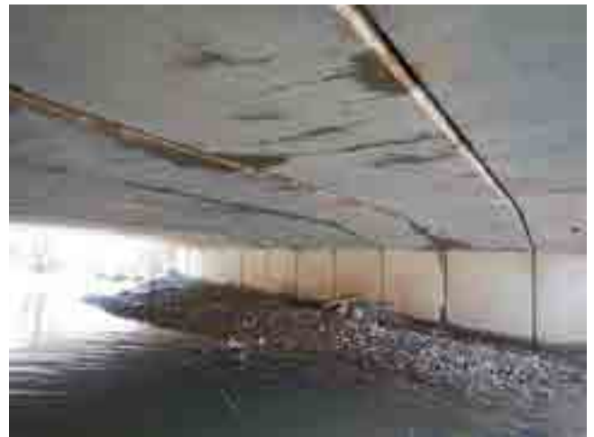
LOOKING WEST AT WATER SEEPAGE BETWEEN PRECAST
