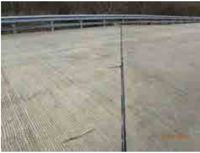
WEST END JOINT SPALL
