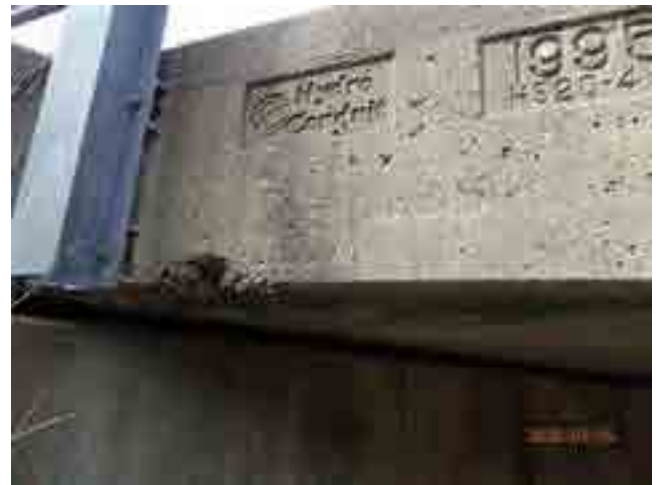
SOUTHWEST BEAM SPALL
