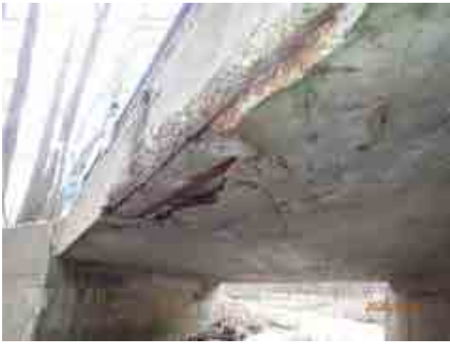
LOOKING SOUTH SPAN REBAR SECTION
