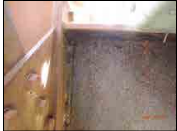
LOOKING AT NORTH TRUSS L6 WITH RUST LAMINATION
