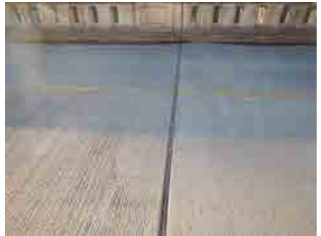
LOOKING AT DIRT FILLED BRIDGE JOINT
