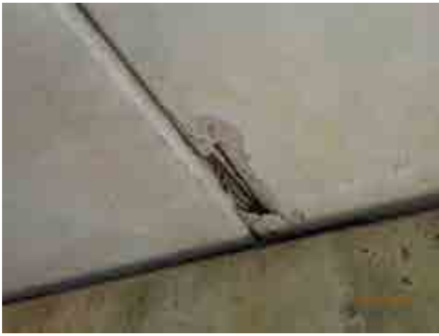
BEAM 4 EAST END SPALL
