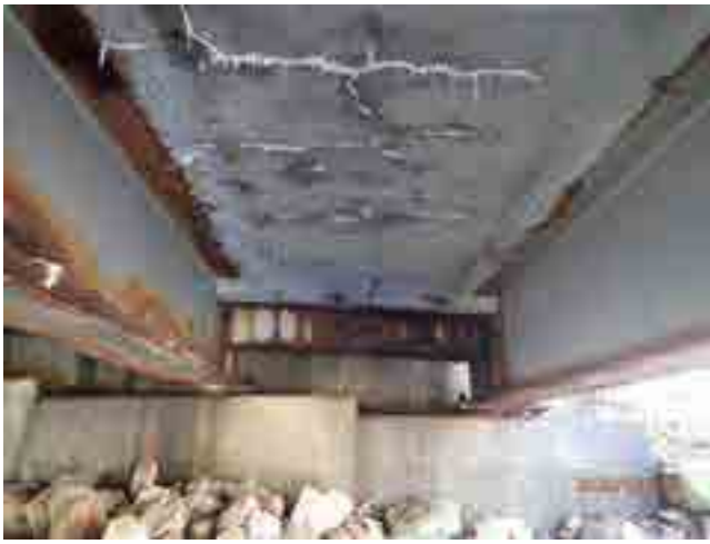
SOUTHWEST CORNER DECK EFFL.
