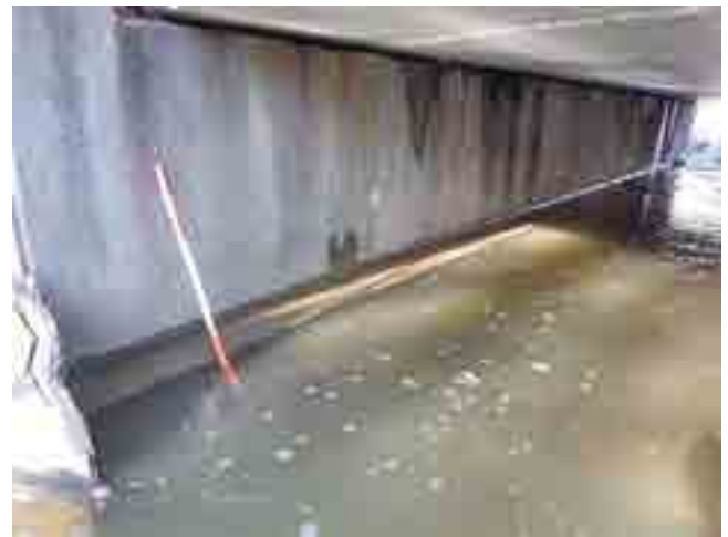
LOOKING EAST AT SCOUR ALONG THE NORTH
