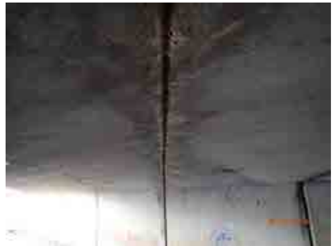
TYPICAL SEEPAGE BETWEEN SEGMENTS
