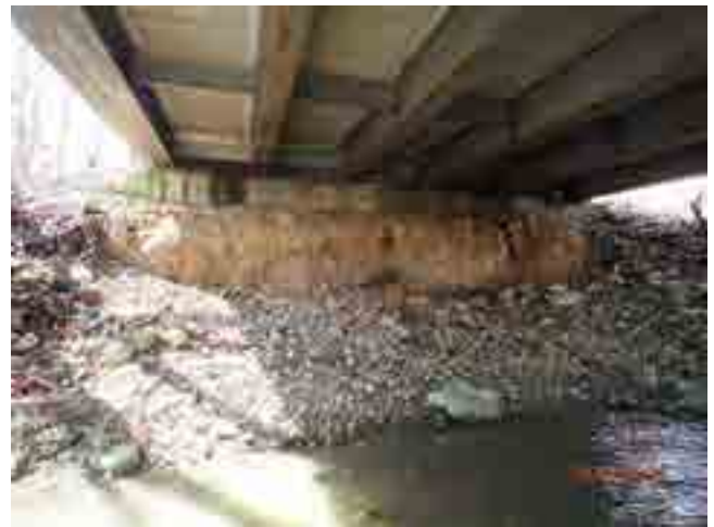
SOUTH ABUTMENT SCOUR
