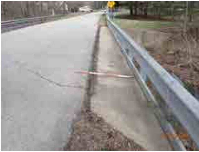
EAST COPING BIT. DROP-OFF
