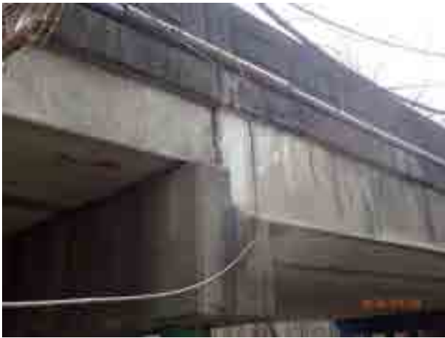
NORTHWEST PIER BEARING EFFL.
