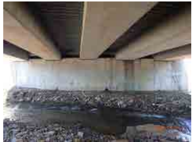
DOWNSTREAM PIER CRACKS AND EFFL.
