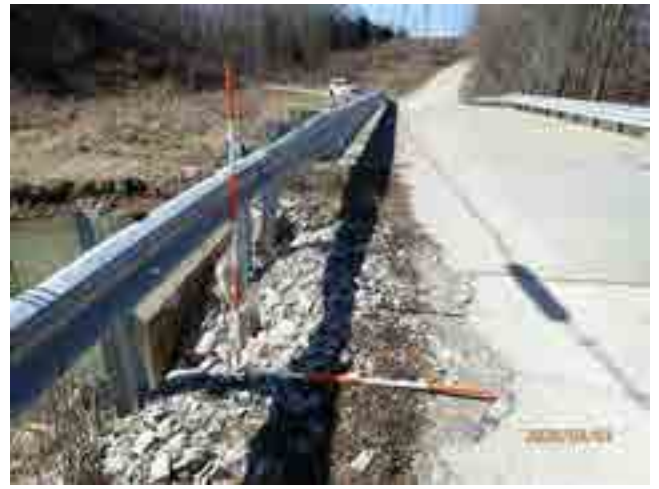
SOUTHEAST CORNER EROSION
