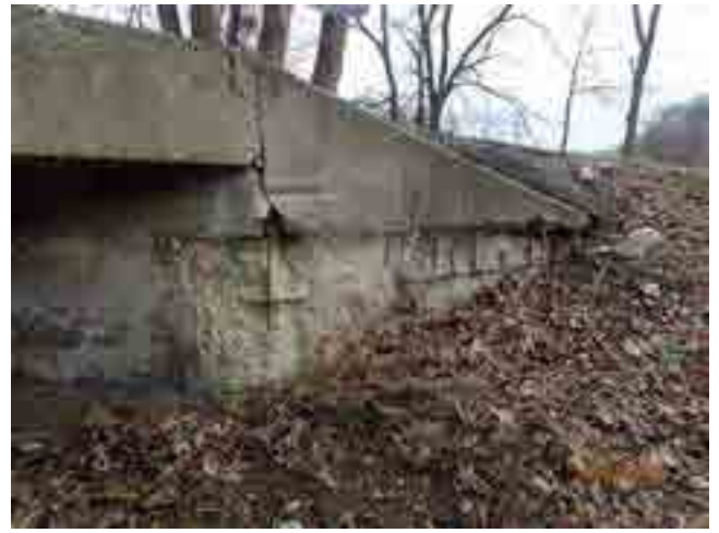
LOOKING SOUTHWEST WING RAVELING
