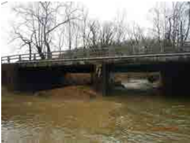
LOOKING EAST AT SILT BUILD-UP IN NORTH SPAN
