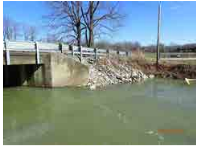
SOUTHEAST CORNER EROSION
