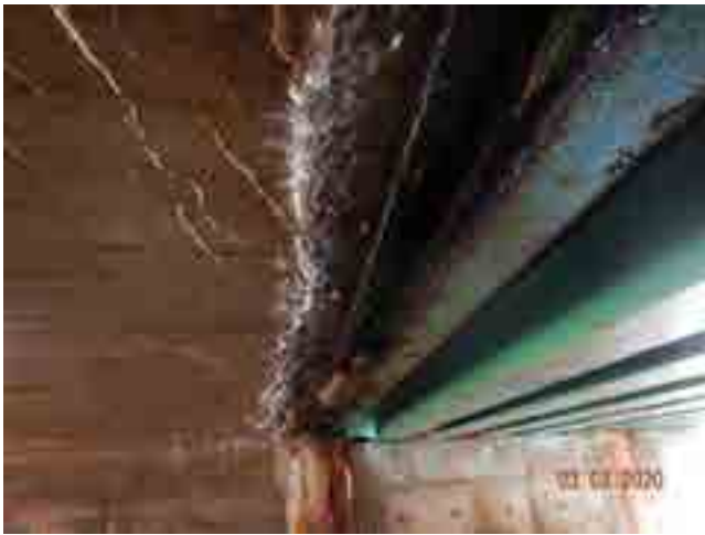
NORTH AT SPALLED SLAB, EXP. RESTEEL, S SPAN
