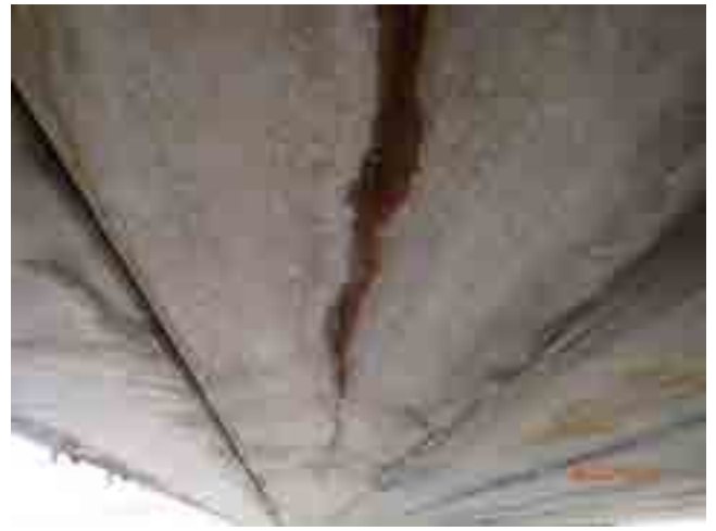
BEAM 2 CRACKS WITH RUST STRAINS
