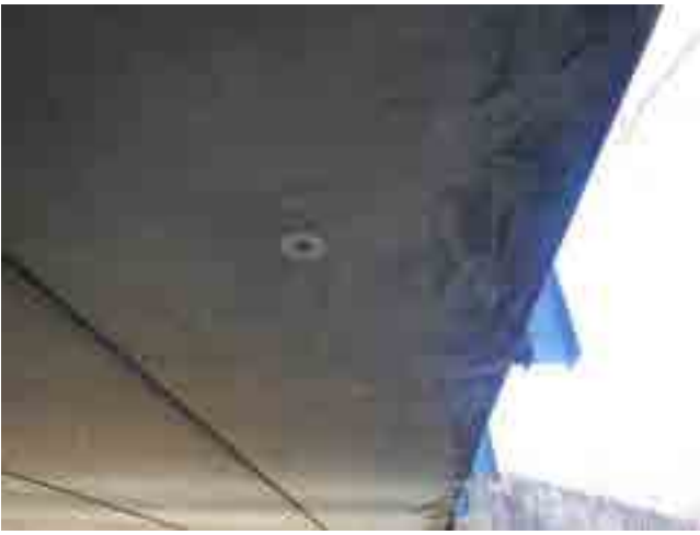
HAIRLINE CRACK ON BOTTOM OF NORTH COPING BEAM
