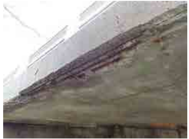
SOUTH SPAN WEST COPING SPALLS
