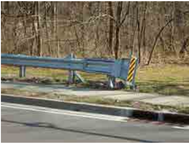
LOOKING SOUTH AT DAMAGED SW GUARDRAIL END
