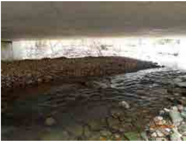
CHANNEL SILT AND VEGETATION BUILDUP
