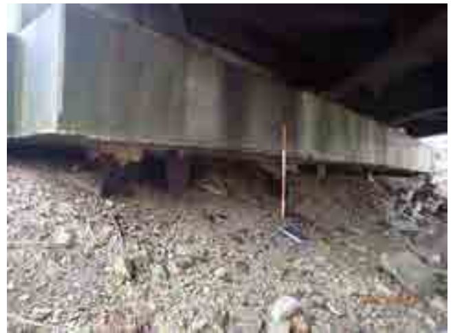
LOOKING EAST AT ABUTMENT SCOUR
