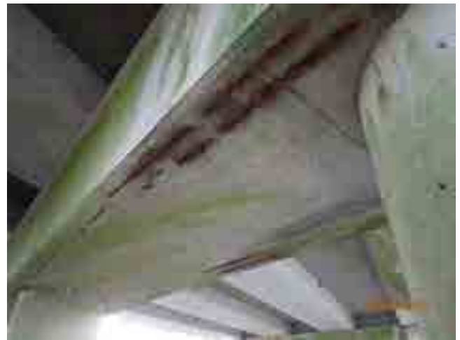
LOOKING EAST AT PIER SPALLS
