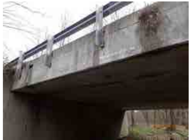
DOWNSTREAM BEAM CRACKS AND EFFL.
