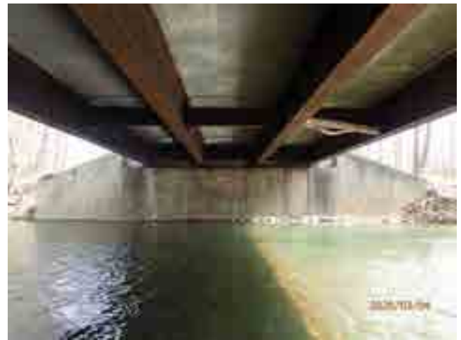
EAST ABUTMENT SCOUR
