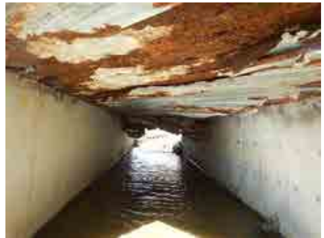
LOOKING WEST AT RUSTED CENTER SPAN METAL
