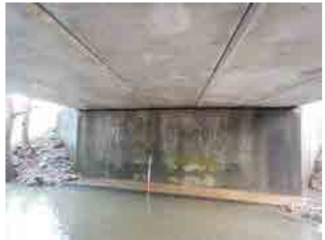
LOOKING NORTH AT NORTH FOOTING EXPOSED
