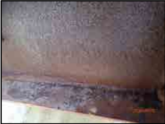
LOOKING AT FLOORBEAM 2 AT FLAKING RUST ON EAST SIDE 1' FROM L2, NORTH TRUSS.
