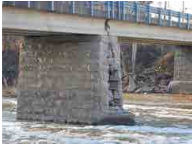
NORTHWEST AT MISSING, DET. OF STONES AT EAST END
