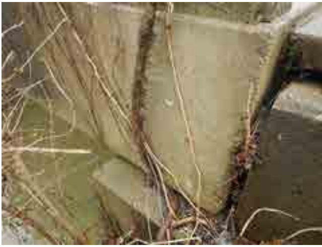
HAIRLINE CRACKS AT SOUTH END OF WEST COPING
