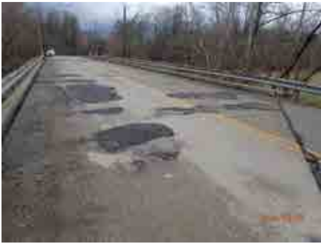
EAST END DECK SPALLS/ PATCHES
