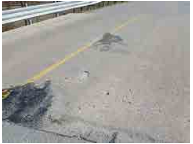
SPALLS, PATCHES, MAP CRACKING ON DECK SURFACE
