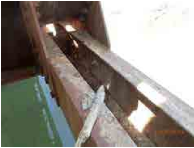
L8-L10, N TRUSS AT FLAKING ON OUTER CH. NEAR L8
