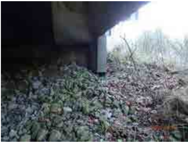
NORTHWEST CORNER EROSION
