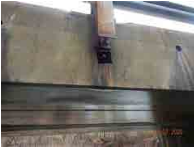
LOOKING EAST AT WEST COPING RUSTED CENTERSPAN
