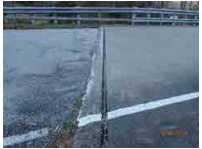
WEST BRIDGE END DAMAGE
