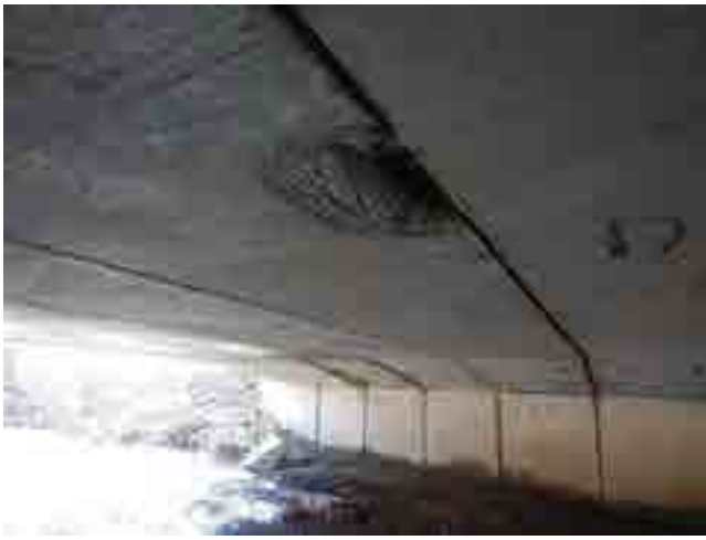
LOOKING WEST AT SPALL IN SECTION
