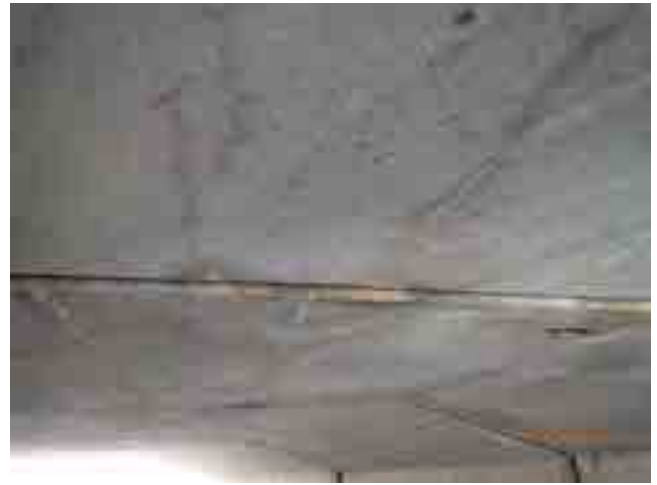
TYPICAL HAIRLINE CRACKS
