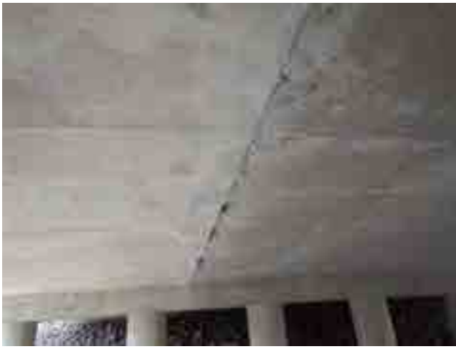
LOOKING SOUTH AT SPALLS, DELAMS. IN CENTER SPAN
