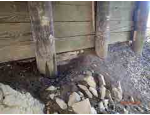
SOUTH ABUTMENT LOSS OF FILL
