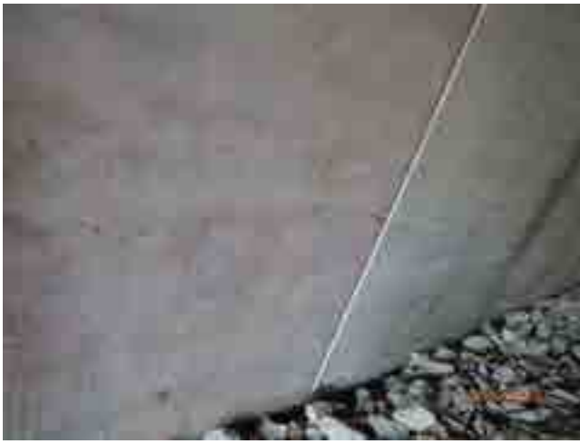
HAIRLINE CRACKS ALONG LEGS
