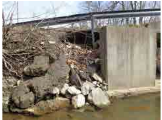
LOOKING NW AT SHOULDER EROSION
