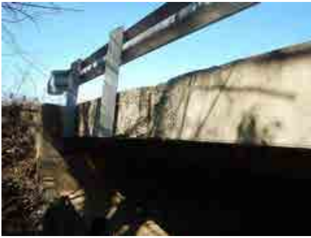
LOOKING SOUTH COPING SPALL
