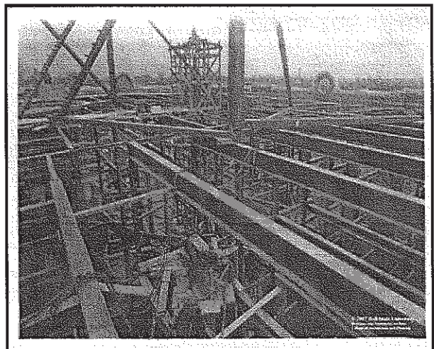
Figure 2, below: Construction photo, looking down from above roof level. Note heavy I-beams and circular framework for the rotunda. The limestone facing has been applied and two of the four clock surrounds are visible on the parapet. Drawings and Documents Archive, Ball State University, 23-18B-007_s_1.
